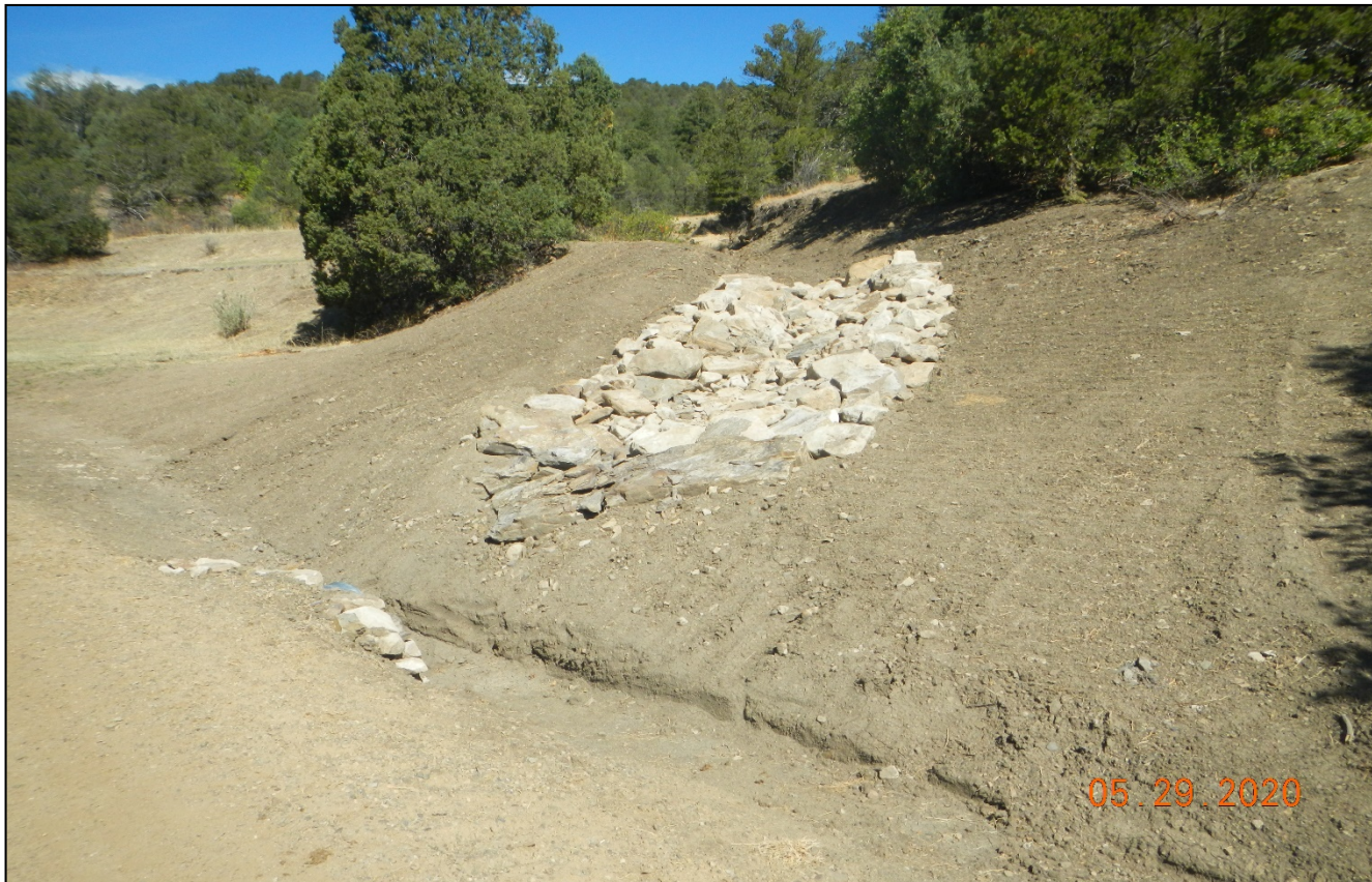
Photo 3. Facing northwest across the road from the location. A berm with rock rip/rap has been installed. Disturbed soils were seeded and tracked.
