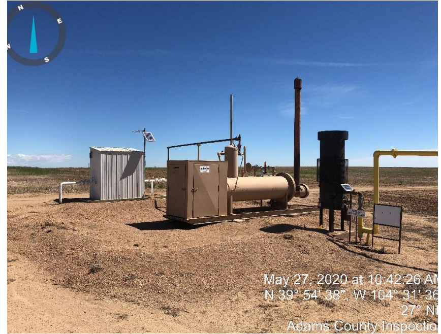
Photo #2 separator, ECD & meter run
