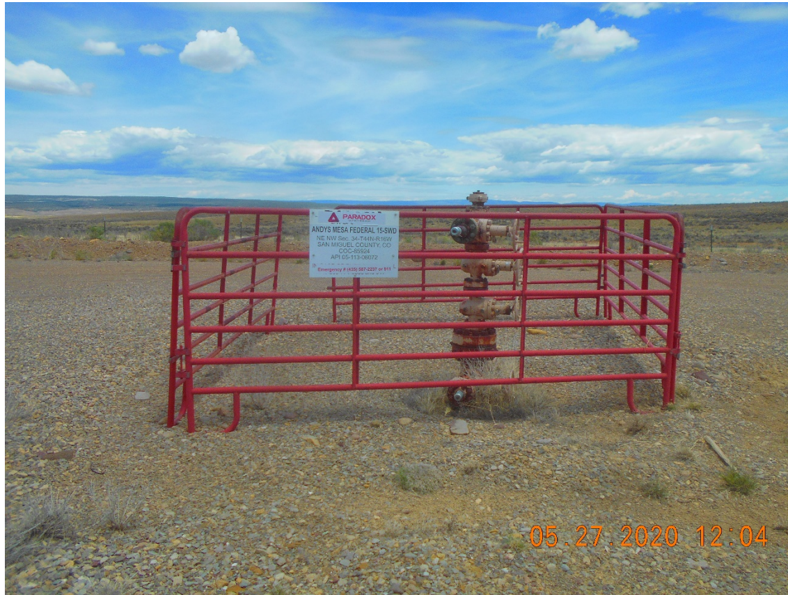
Injection Wellhead – Temporarily Abandoned
