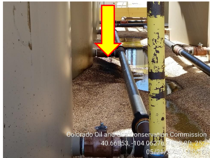
Photo 6 – Stained Soil at South Middle-East Loadline
