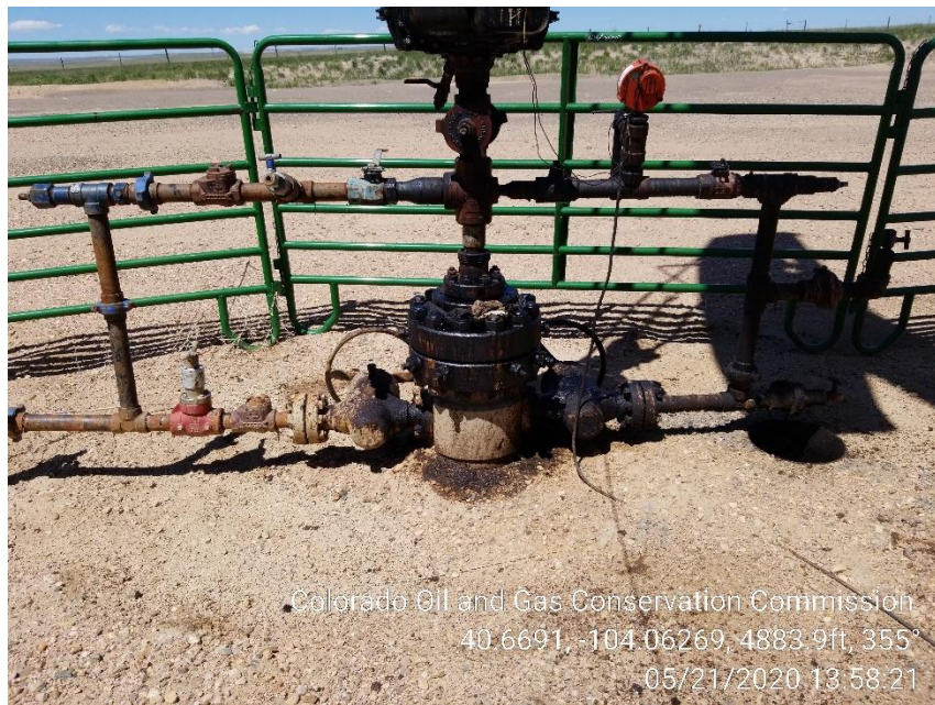
Photo 5 – Stained Soil at 1-14-8-60 Wellhead
