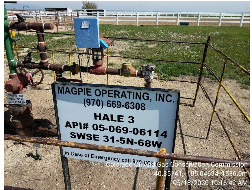
Wellhead sign on 5/18/2020
