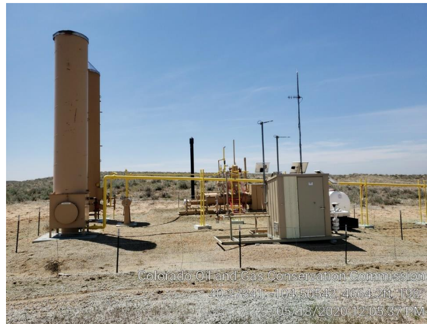
Photo #2 Separator, ECD's & Meter Runs
