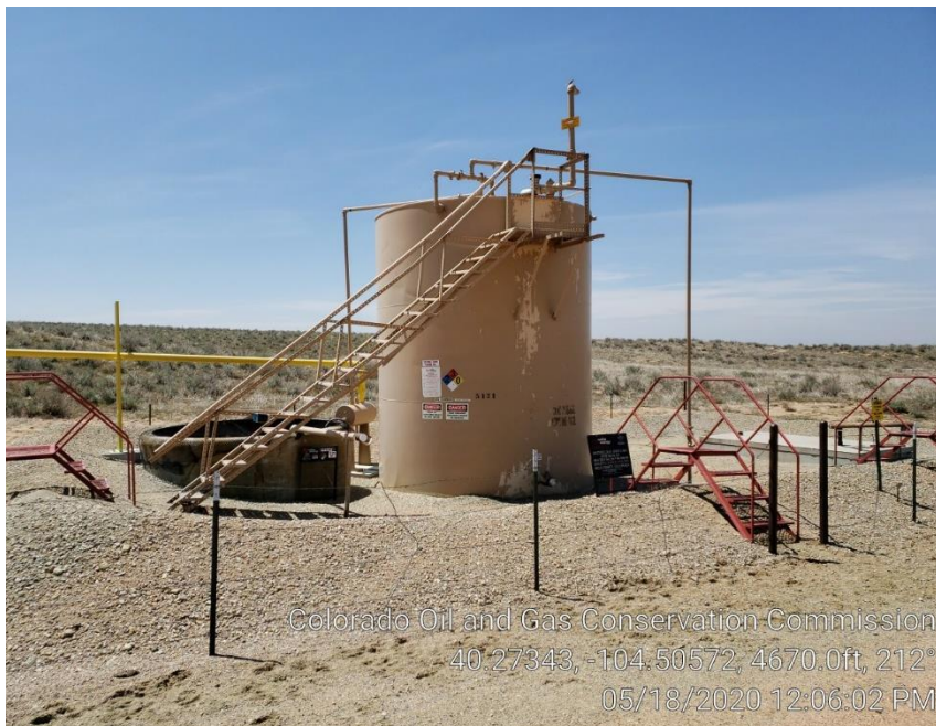
Photo #3 Tank Battery
