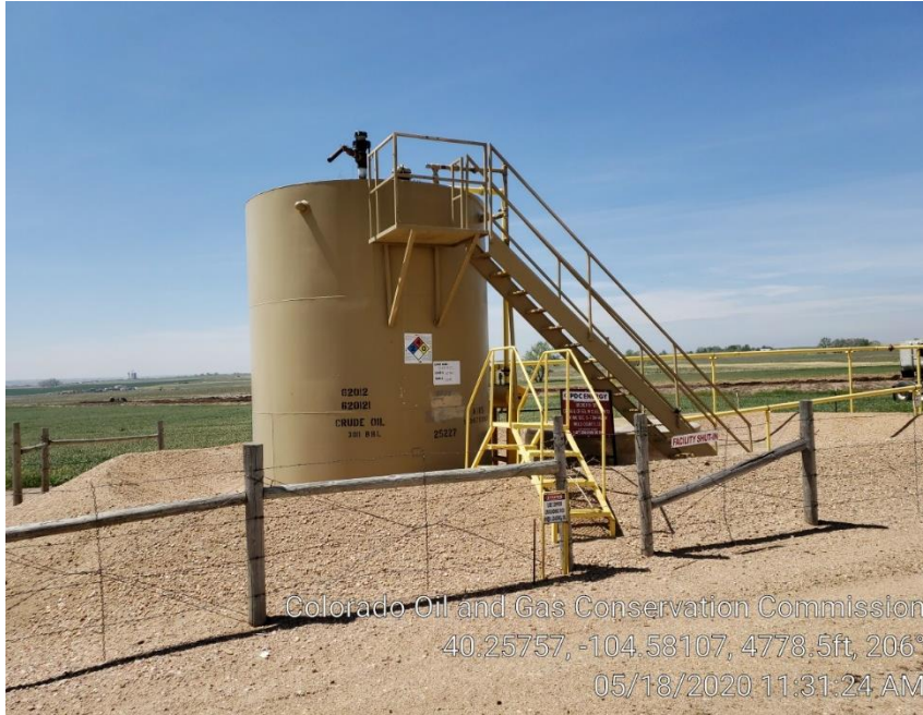
Photo #2 Tank Battery
