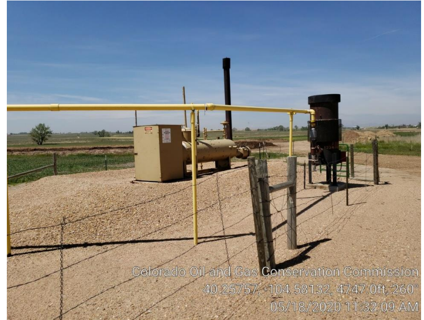
Photo #3 Separator & ECD
