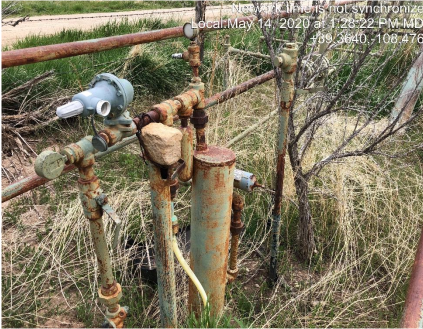
Photo #1192 Domestic tap off of sales line.
