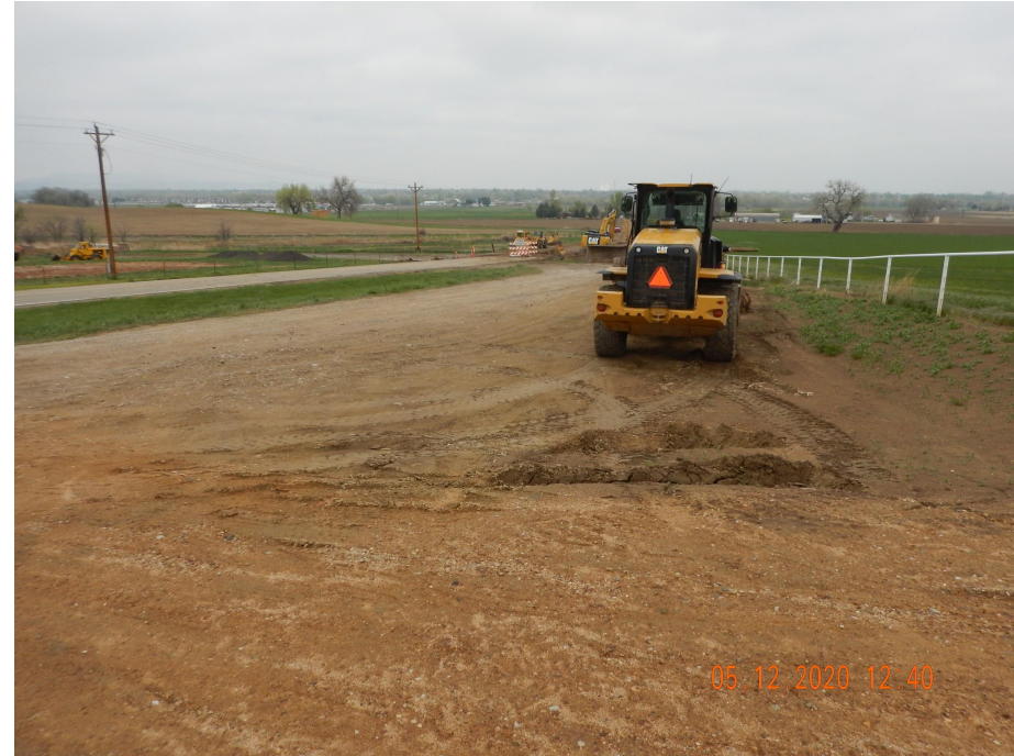
Photo 9. Photo taken from the other portion of the associated offsite tank battery location, facing North. Photo illustrates location is currently being used as a construction staging area for a new sewage installation.
