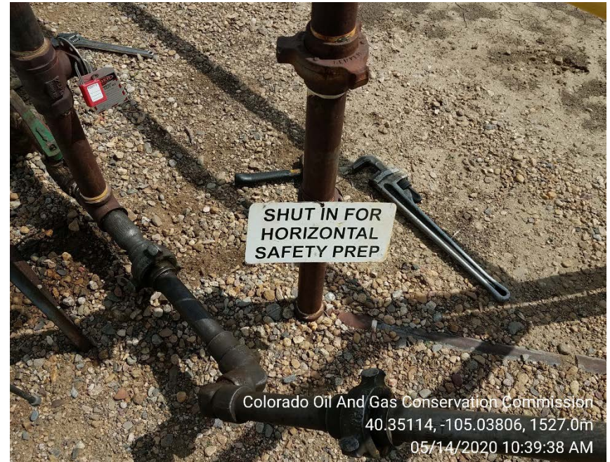
HZ safety prep sign
