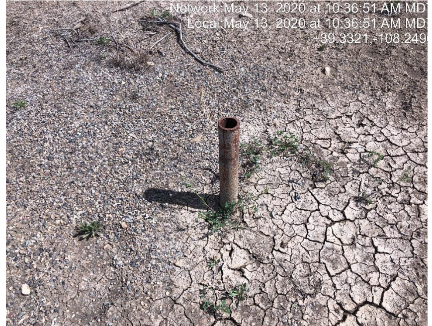
Photo #1170 Flow line riser not LO/TO.
