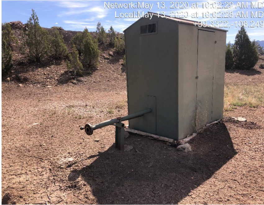
Photo #1166 Unused meter run.
