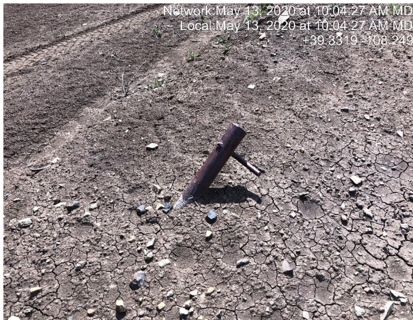
Photo #1169 Multiple unmarked deadman.
