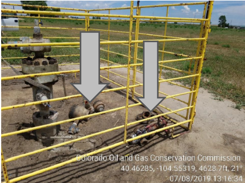
Photo #9 Ankeney 2-28 Wellsite Unused Equipment (well parts) prior insp.
