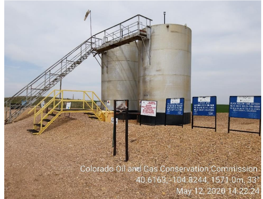
Photo 2: Crude oil tanks
