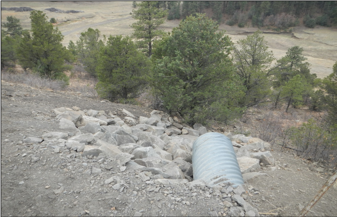
Photo 3. Culvert outlet protection has been installed on some of the culverts leading to the location.
