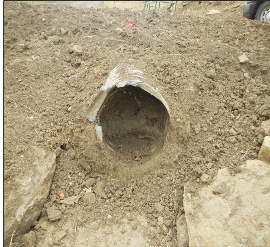
Photo 2. The culvert was observed to be full of sediment on both ends. This culvert will likely need to be replaced.
