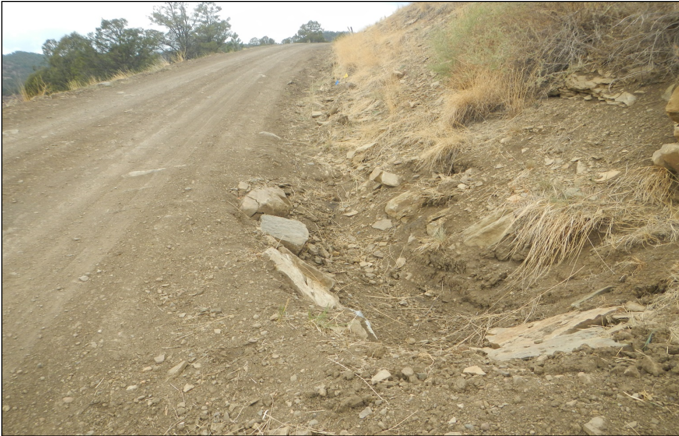
Photo 3. The culvert inlets along the road leading to the location have been repaired.
