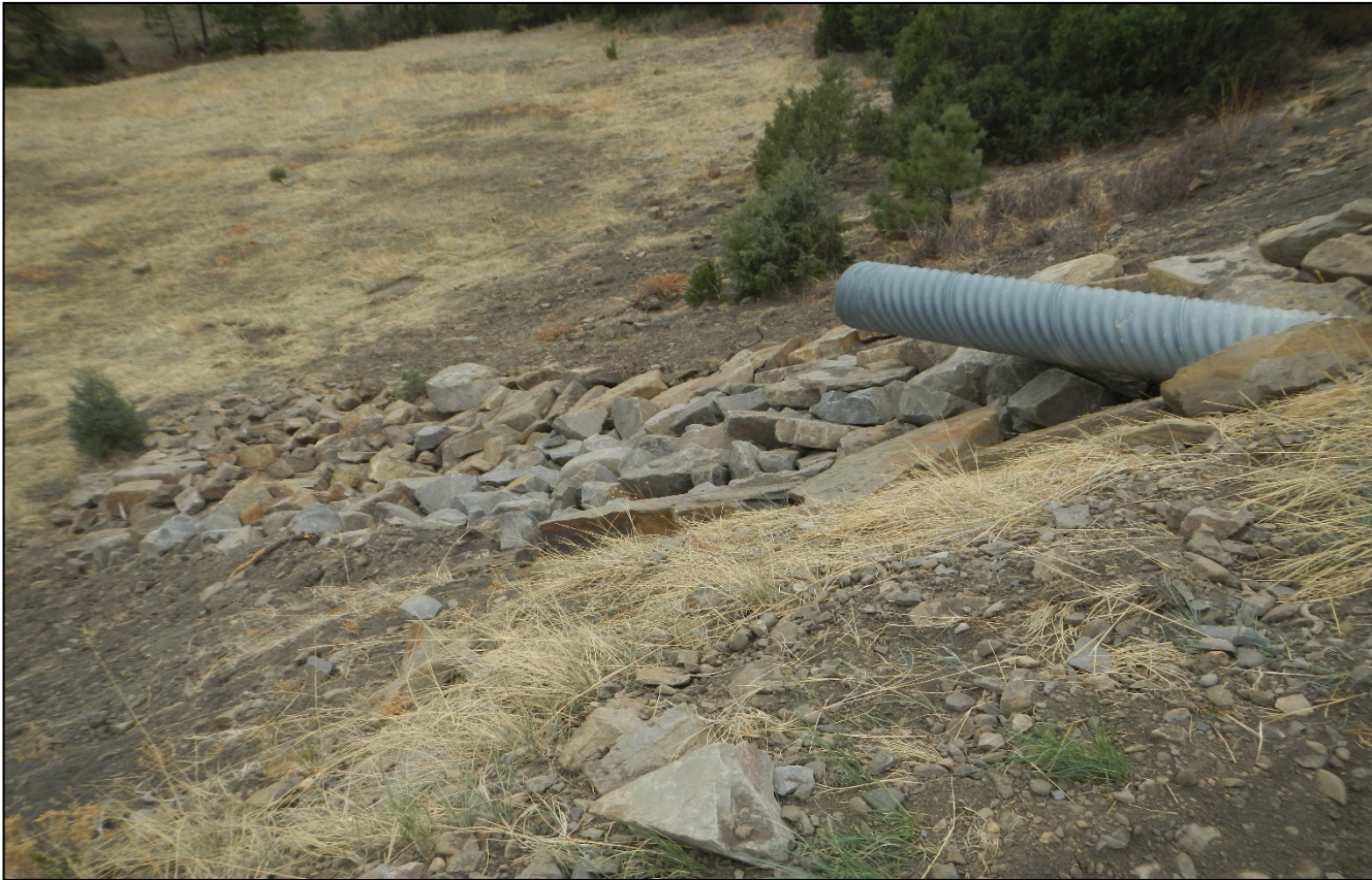
Photo 2. Outlet protection has been installed on some of the culverts leading to the location.
