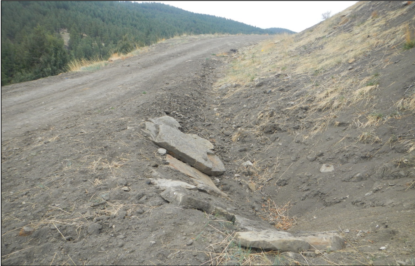
Photo 1. The culvert inlets along the road leading to the location have been repaired.
