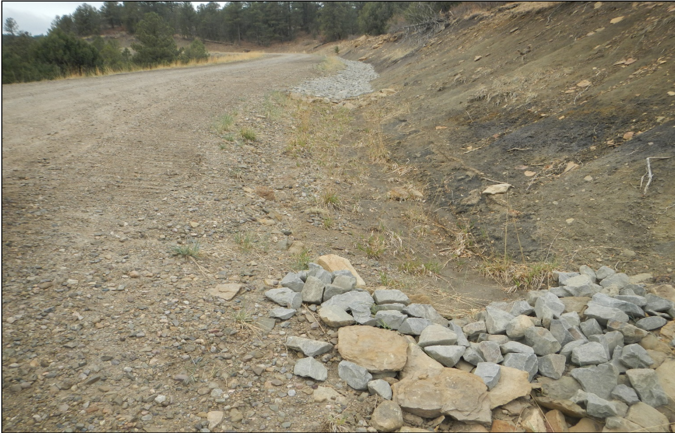
Photo 3. Additional rock rip/rap and check dams have been installed along the side of the road to prevent erosion.
