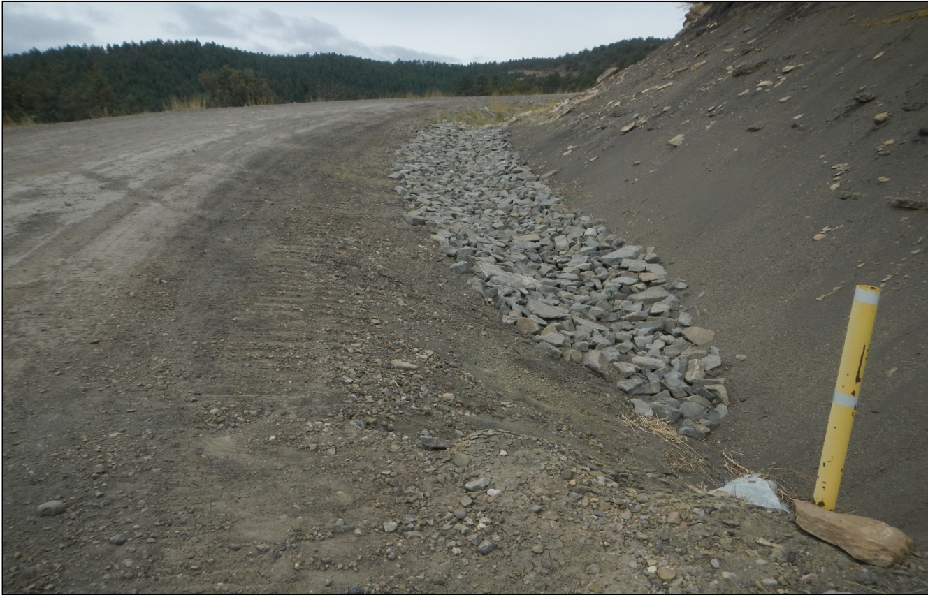
Photo 4. Rock rip/rap has been installed along the side of the road to prevent erosion. The culvert has been maintained and sediment cleaned out.
