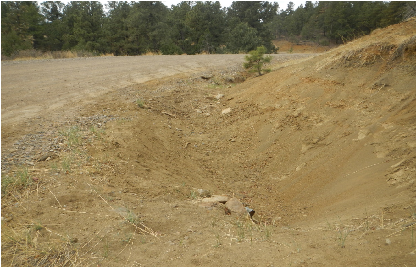
Photo 8. This culvert along the main road has filled in with sediment.
