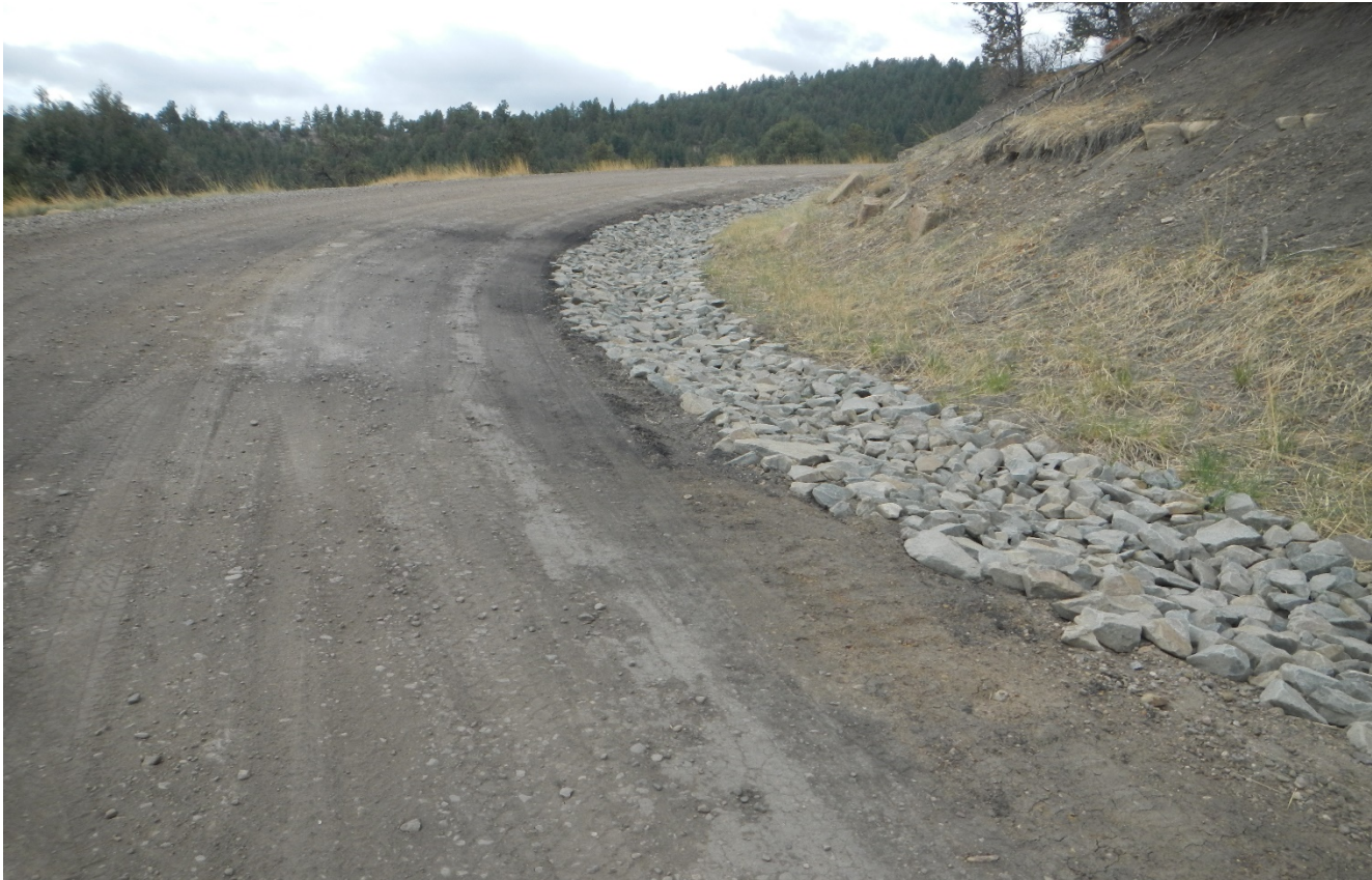
Photo 5. Further up the main road. Rock rip/rap has been installed along the side of the road to prevent erosion.
