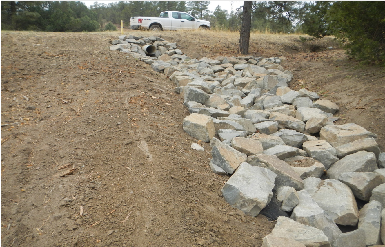
Photo 2. Further up the road, outlet protection has been installed where erosion was during previous inspection.
