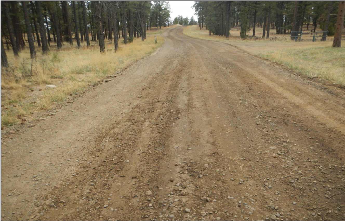
Photo 1. Facing southwest along the main road. The road has been graded and maintained.
