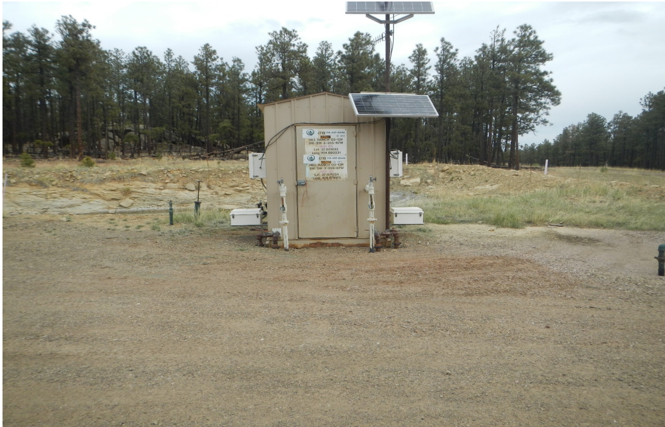
Photo 5. The well sign is posted at the meter shed.
