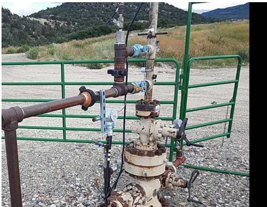
Unmarked well head
