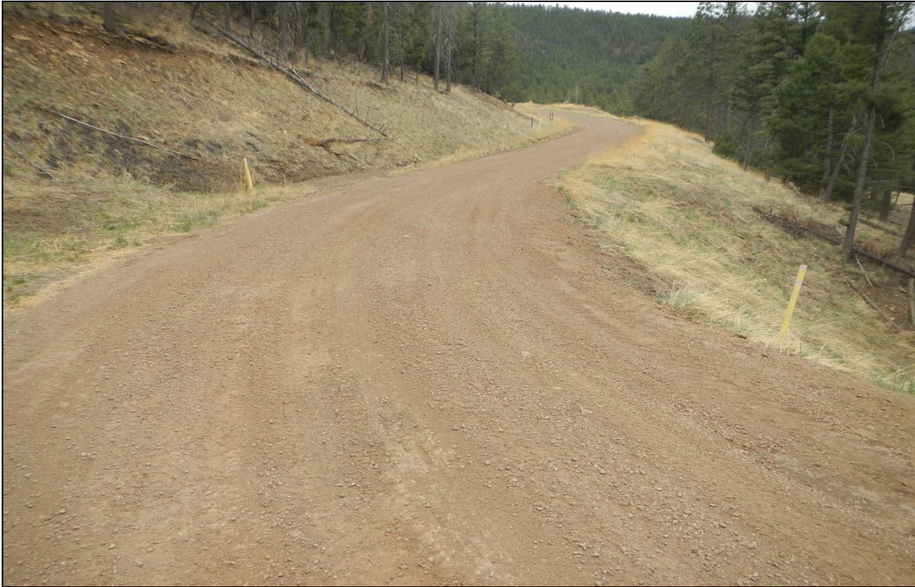
Photo 3. The culvert inlet has been maintained and erosion repaired along the road.
