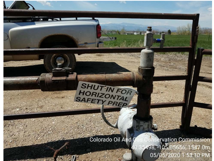
HZ safety prep sign
