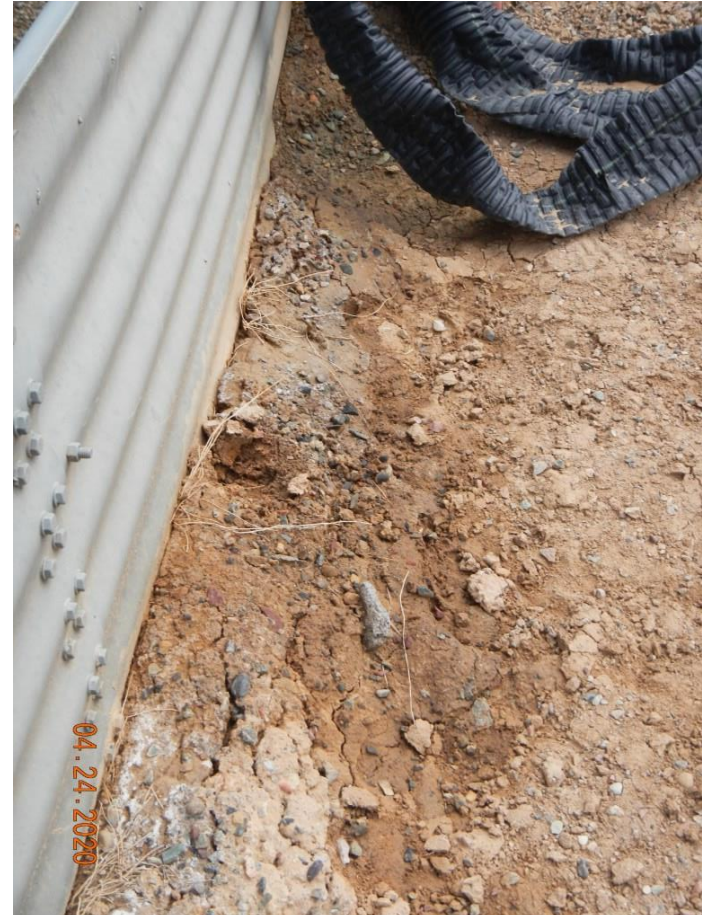
Photo#5: Check to determine if Liner leaking.
