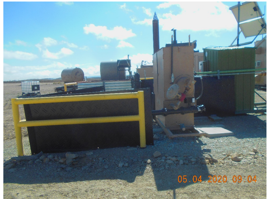
Separator and meter housing
