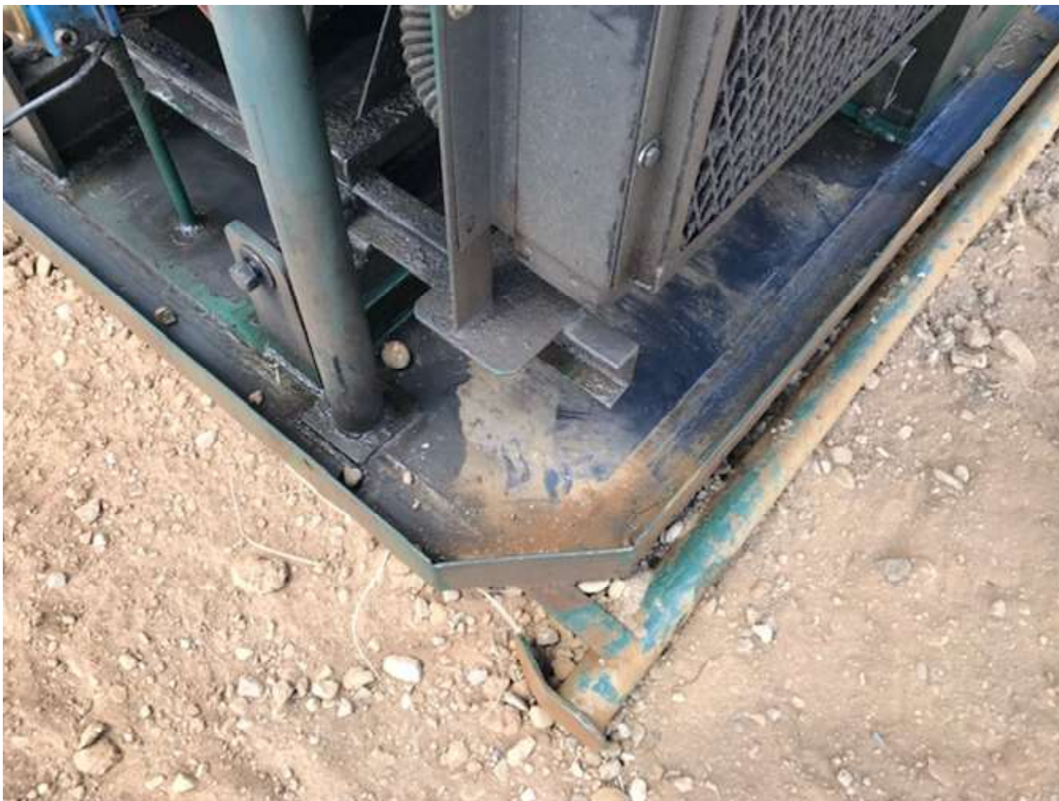
PHOTO 1: THE FLUID ACCUMULATION WAS REMOVED FROM THE LIQUID RING COMPRESSOR CONTAINMENT SKID.
