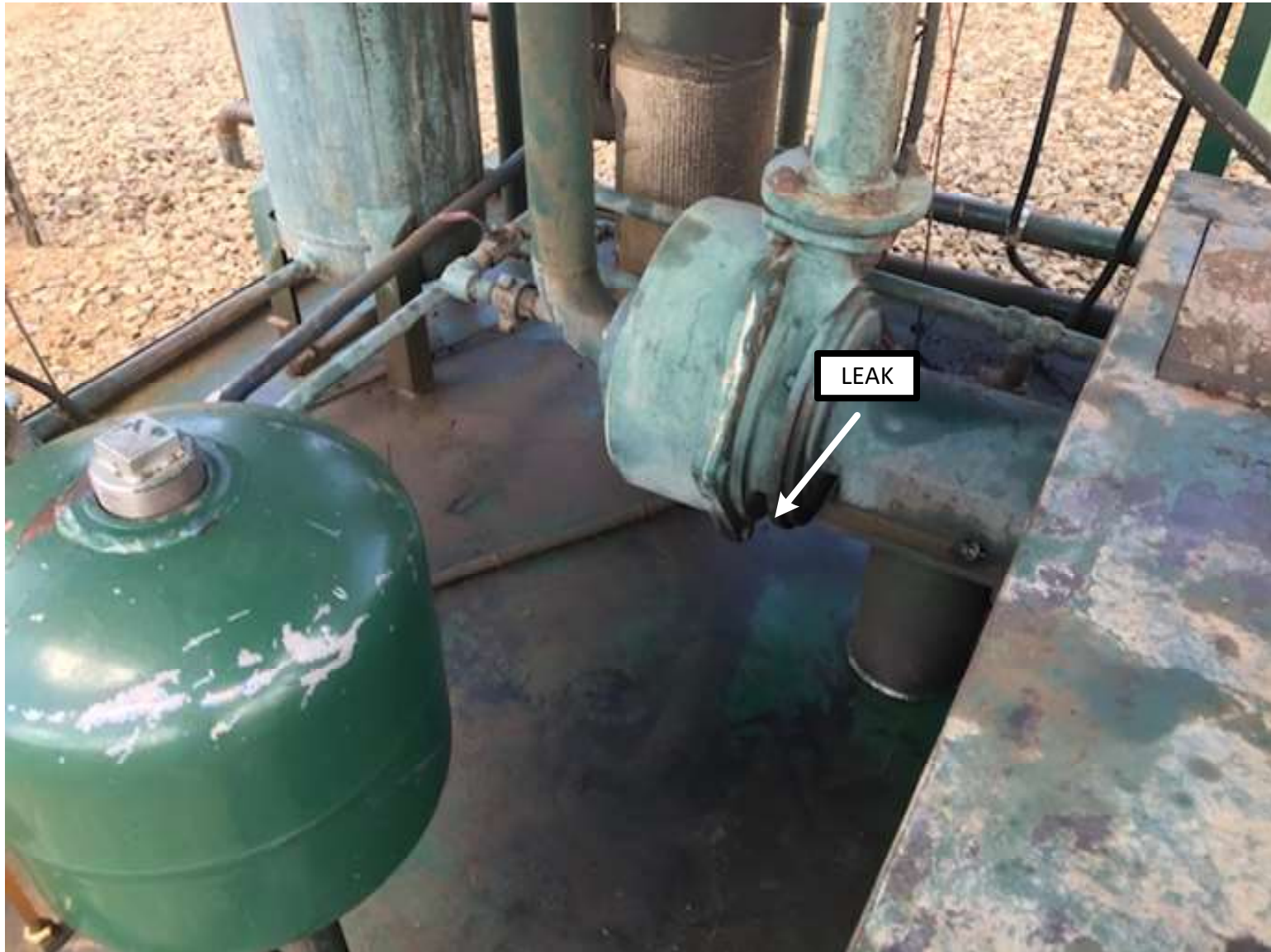
PHOTO 4: THE LEAK ON THE LIQUID RING COMPRESSOR WAS REPAIRED AND THE CONTAINMENT WAS CLEANED UP.
