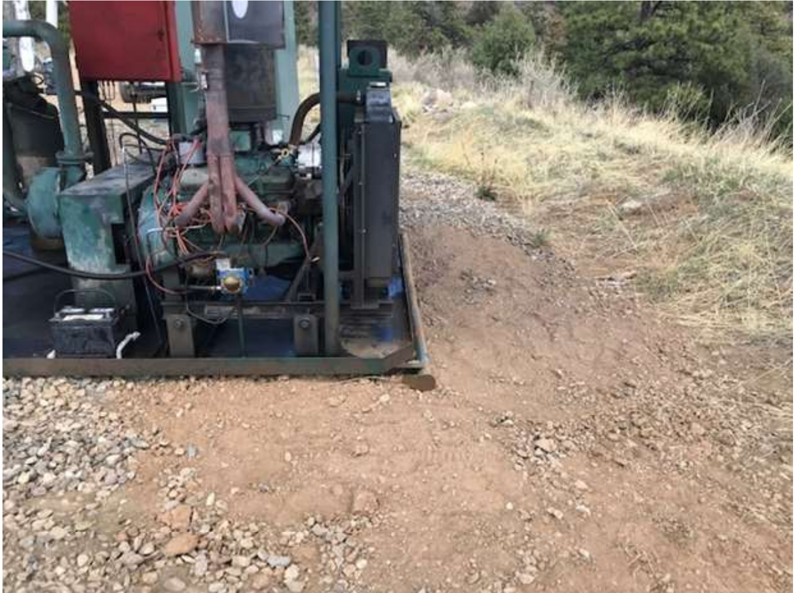
PHOTO 2: THE IMPACTED SOIL/GRAVEL NEAR THE LIQUID RING COMPRESSOR WAS REMOVED AND THE LEAK WAS REPAIRED.
