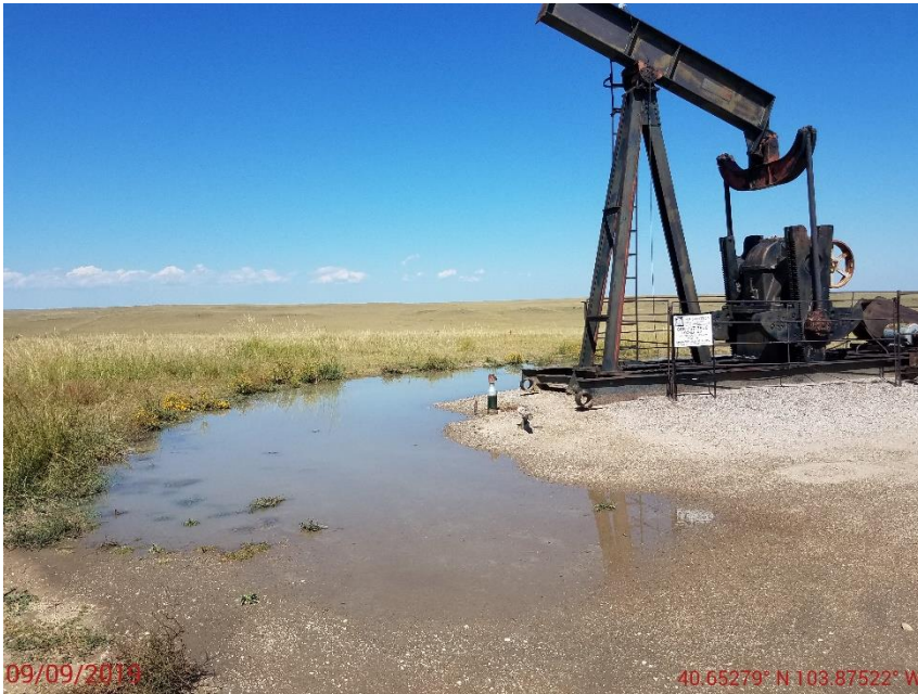
Photo 1: Photo taken from the north end of the location, facing south. Photo shows stormwater ponding around well and location.
