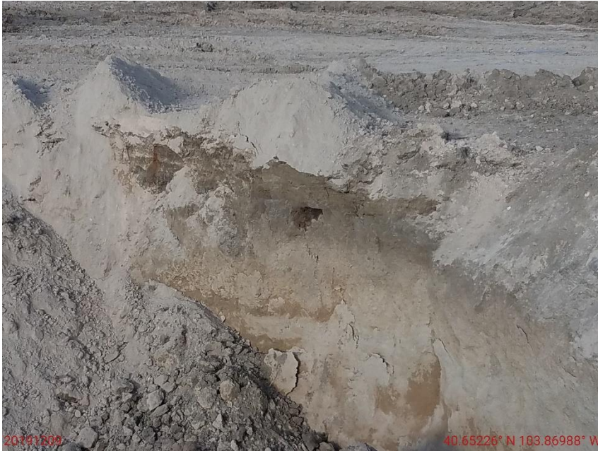
Photo 5: Photo of the excavated area on the east end of the location. Photo shows soils on location.
