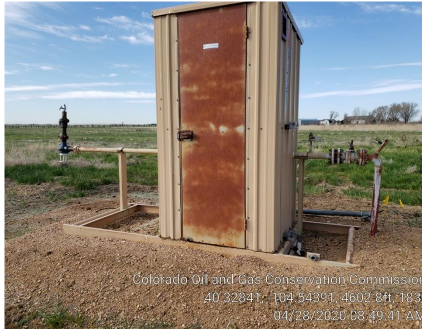
Photo #3 Meter Run
