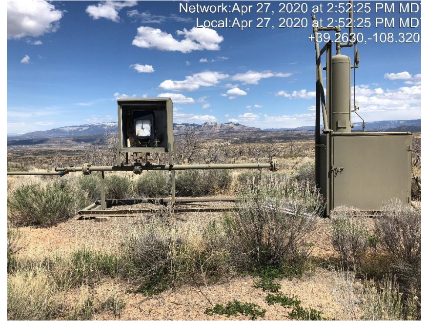
Photo #1077 Multiple places with unused equipment on location.
