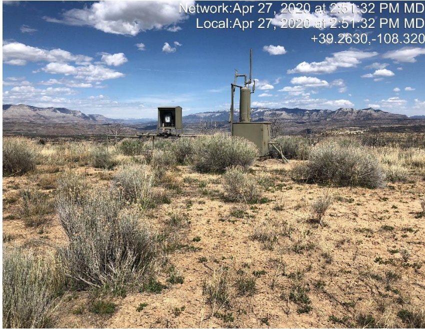
Photo #1074 Multiple places with debris on location
