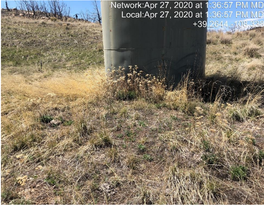
Photo #1066 Multiple places with debris on location.
