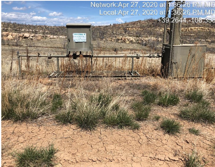
Photo #1064 Multiple places with debris on location.
