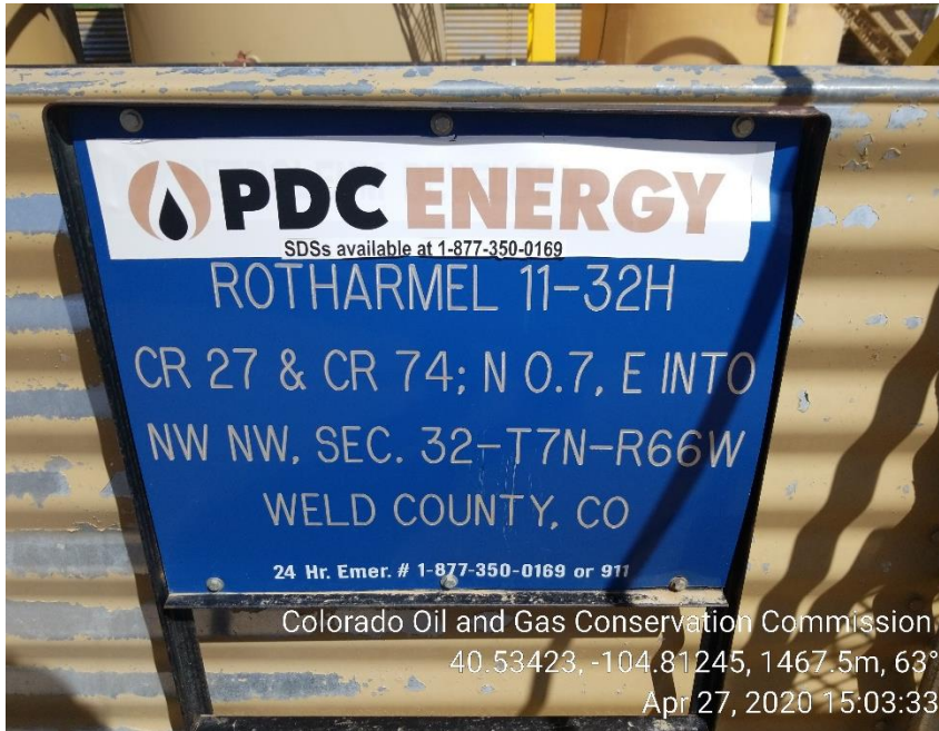
Photo 1: Tank Battery Sign
