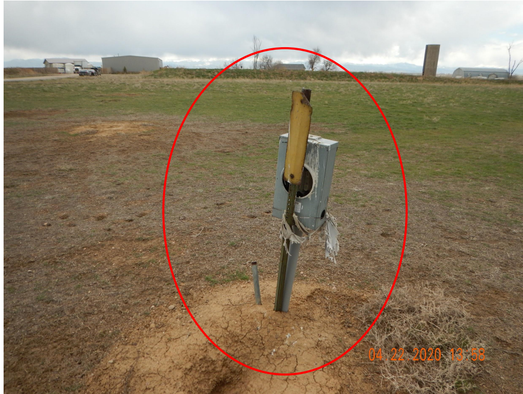
Photo 1. Photo taken from the location of the former AMOCO-CHARTER-SCHNEIDER #1 well, facing West. Operator shall remove all remaining equipment per Rule 1004.a.
