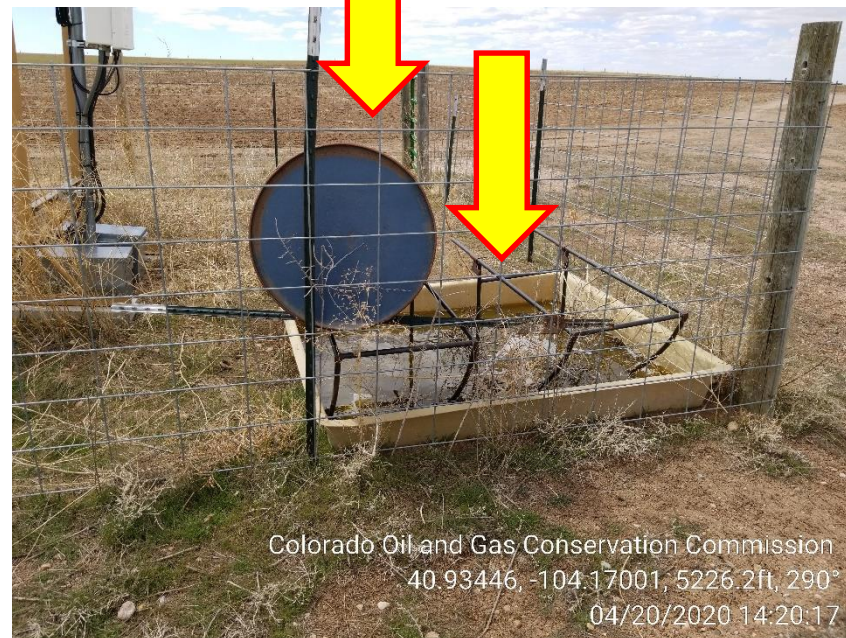
Photo 4 – Unused Chemical Tank, stands and Secondary Containment
