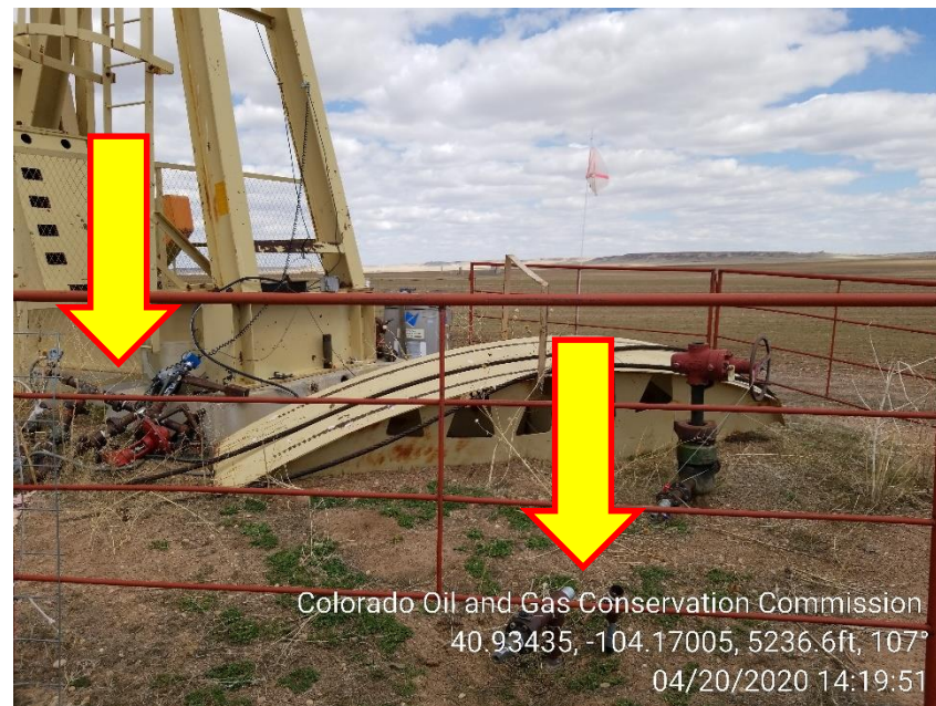
Photo 2 – Unmarked Risers, Unused Wellhead parts
