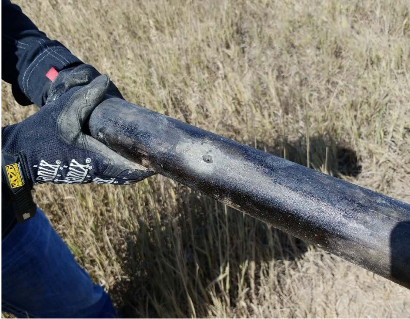
Failed section of pipe.
