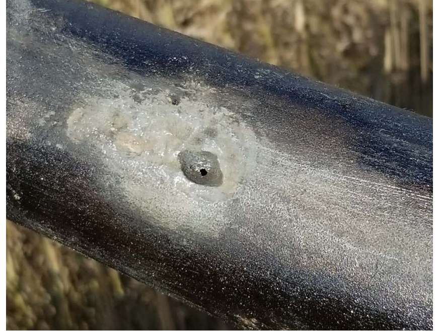
Failed section of pipe
