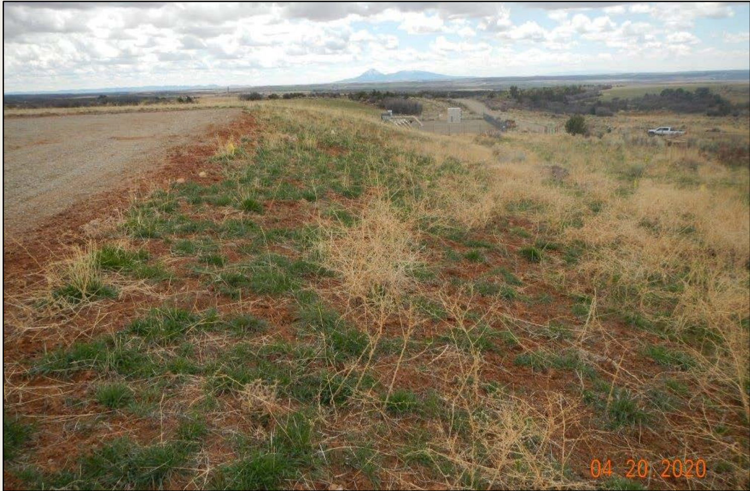
Photo 3. View of the western fill slope from the northwestern edge facing southward.
