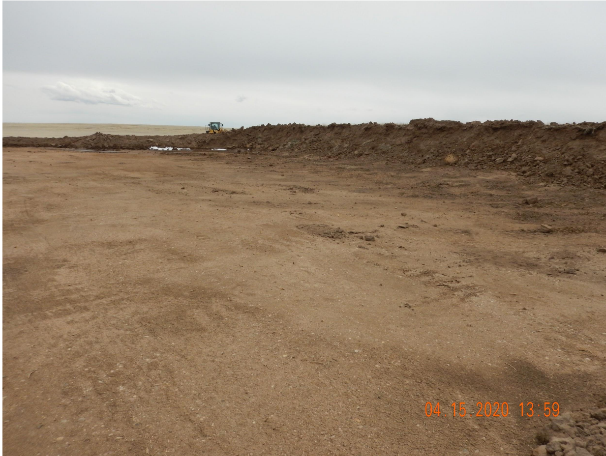
Photo 2. Photo taken from the northern location, facing South. See comments under Photo 1. Appears the Operator is starting to spread topsoil. Operator shall cross-rip disturbance areas to a depth of 18" prior to spreading topsoil. Note: There is a ditch and berm around the downgradient perimeter of location.
