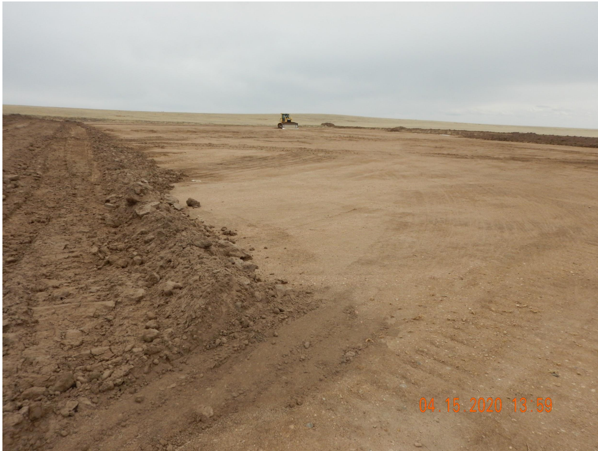
Photo 3. Photo taken from the northern location, facing East. See comments under Photo 1 and 2.
