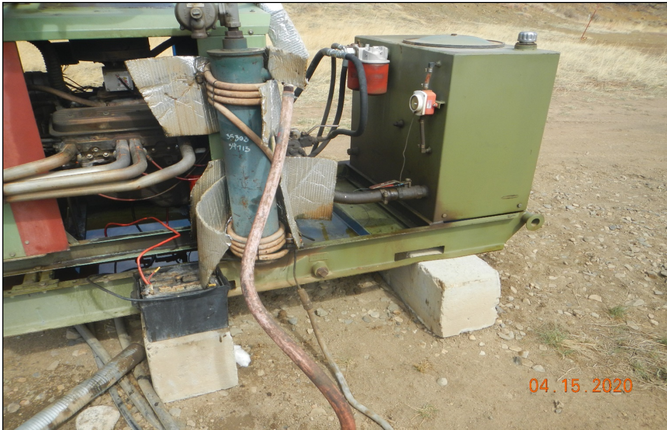
Photo 3. The oily waste on engine skid has been cleaned up.
