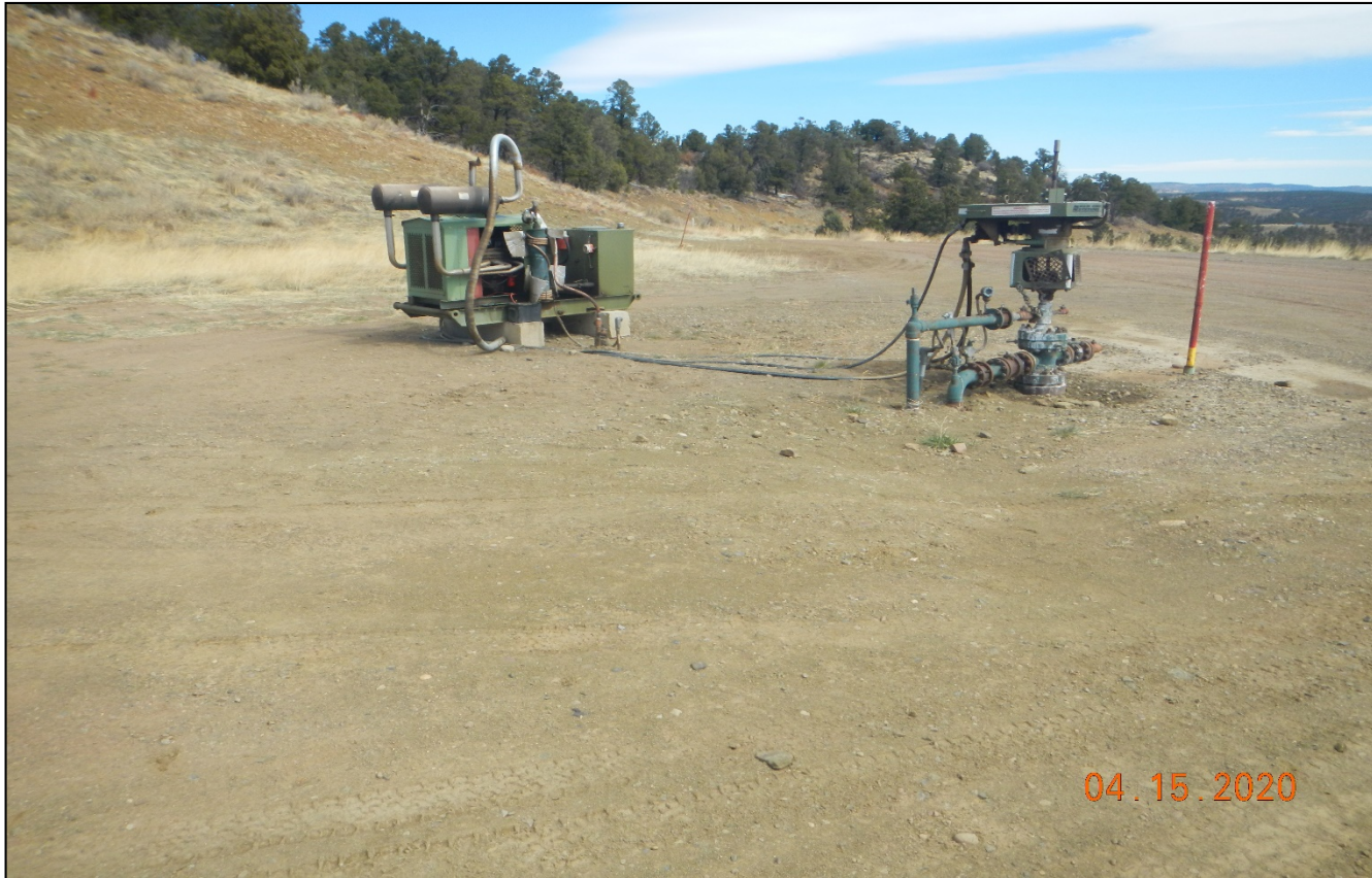
Photo 2. The dripping water leak at the wellhead has been stopped.
