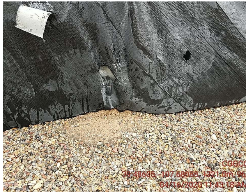
holes in containment
