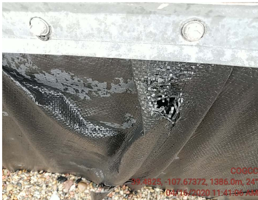
holes in containment
