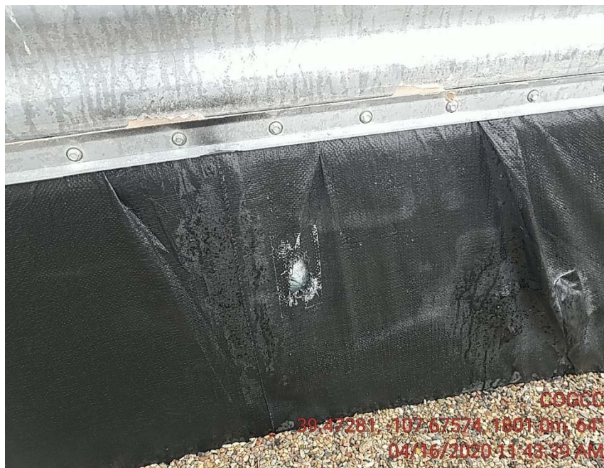
holes in containment
