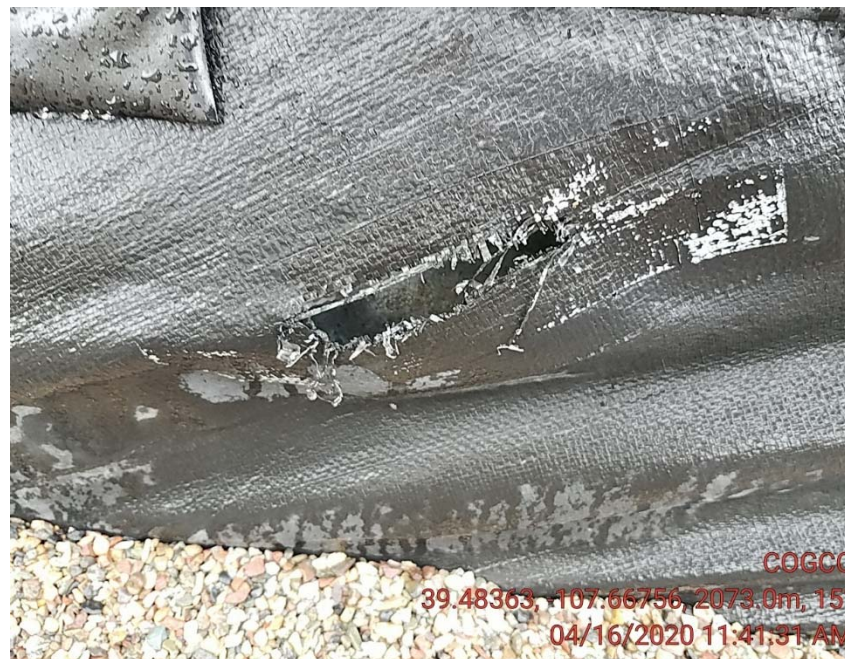
holes in containment
