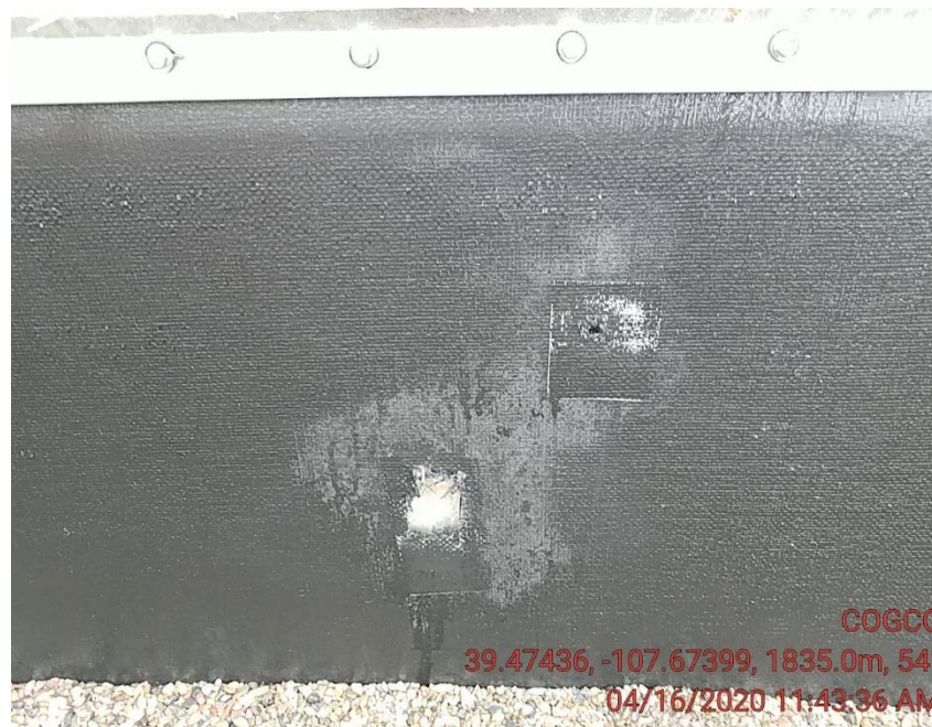
holes in containment
