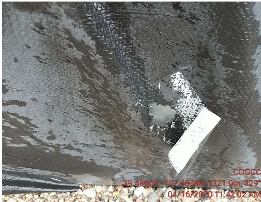
holes in containment
