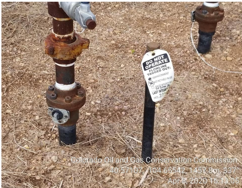
Photo 3: LO/TO riser (for future use)
