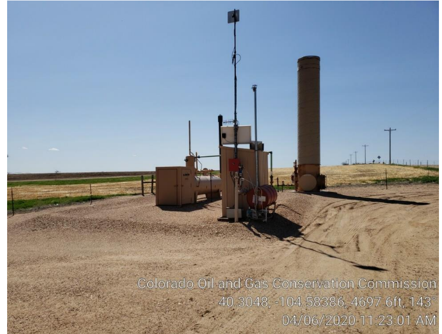
Photo #4 Separator, ECD & Meter Run
