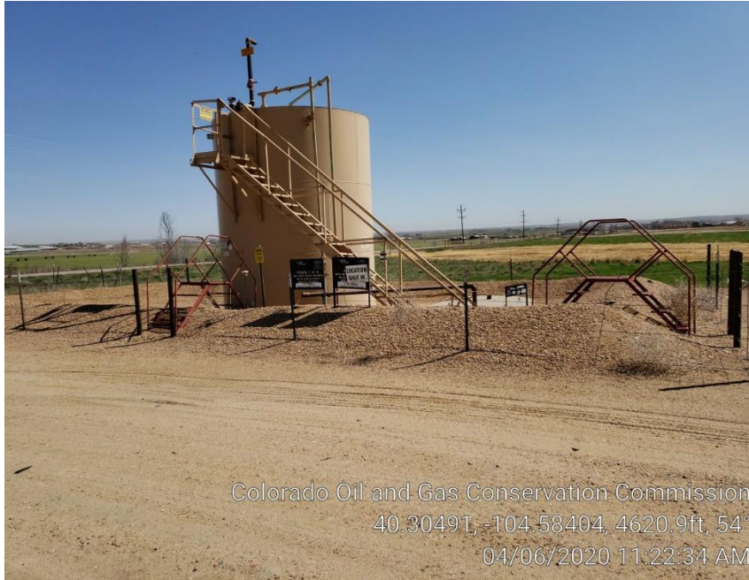
Photo #3 Tank Battery
