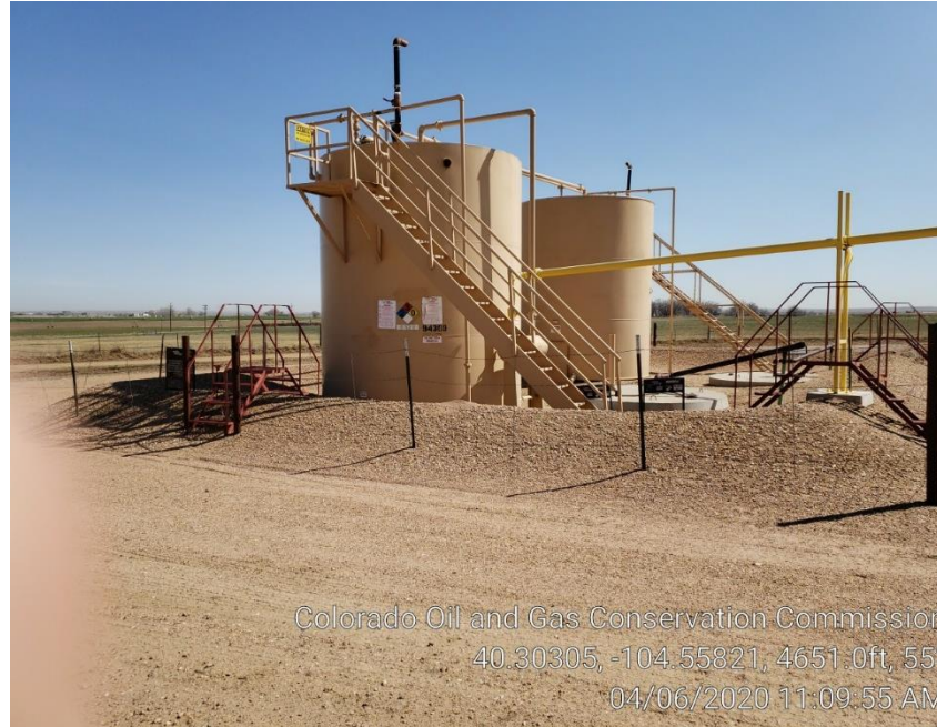
Photo #3 Tank Battery
