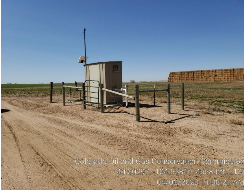
Photo #1 Meter Run
