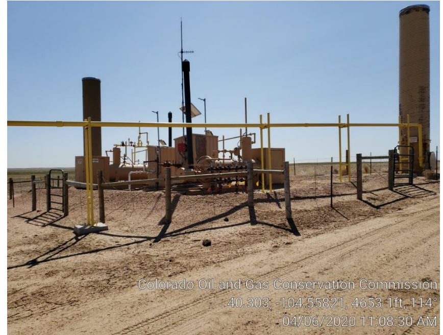
Photo #2 Separators, ECD's & Meter Runs
