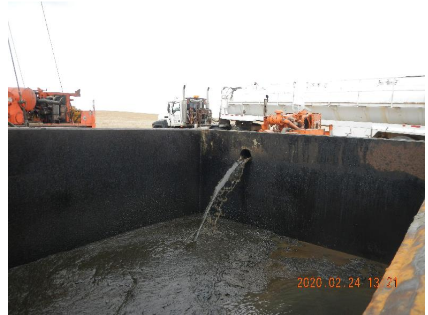
Photo 6: Returns to tank from well.
