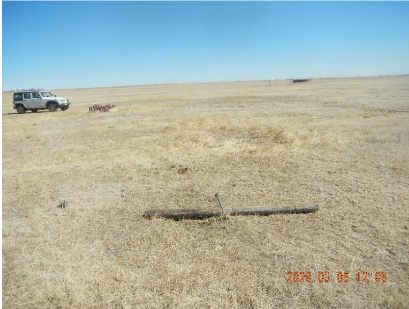
Photo 3: 1" flow line at wood post looking towards header.
