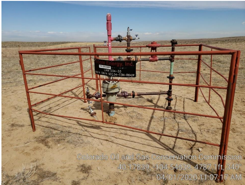
Photo #1 Well & Sign
