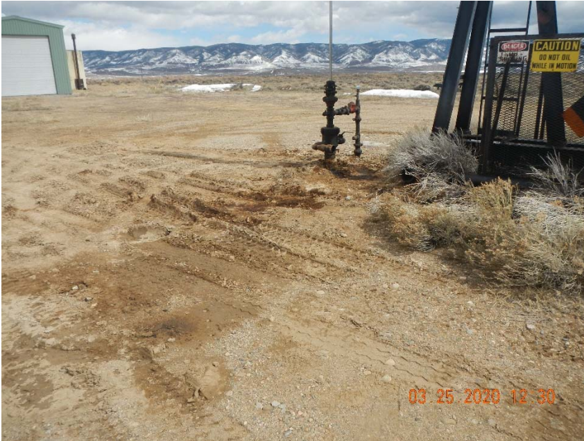
Photo 3. Stained soil at wellhead.
