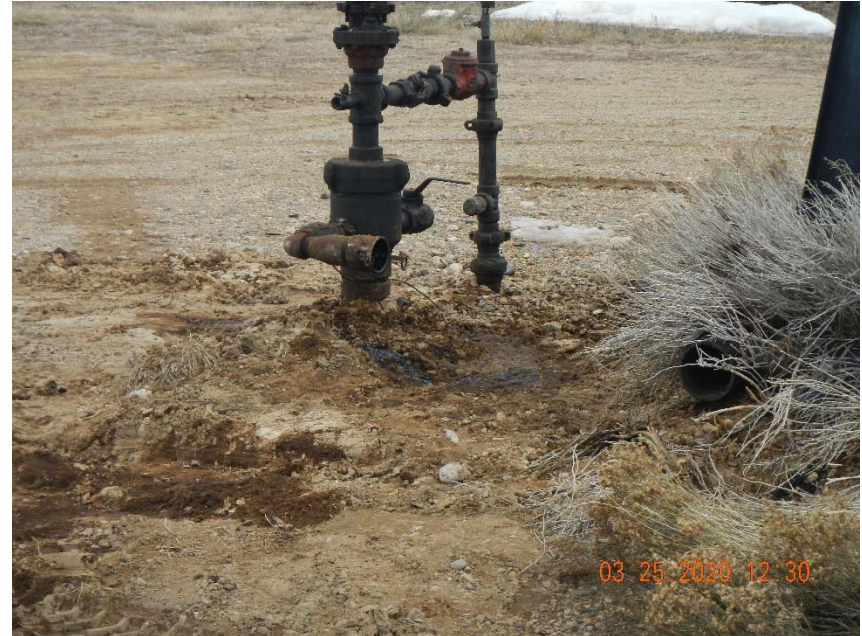
Photo 4. Close-up of stained soil at wellhead.
