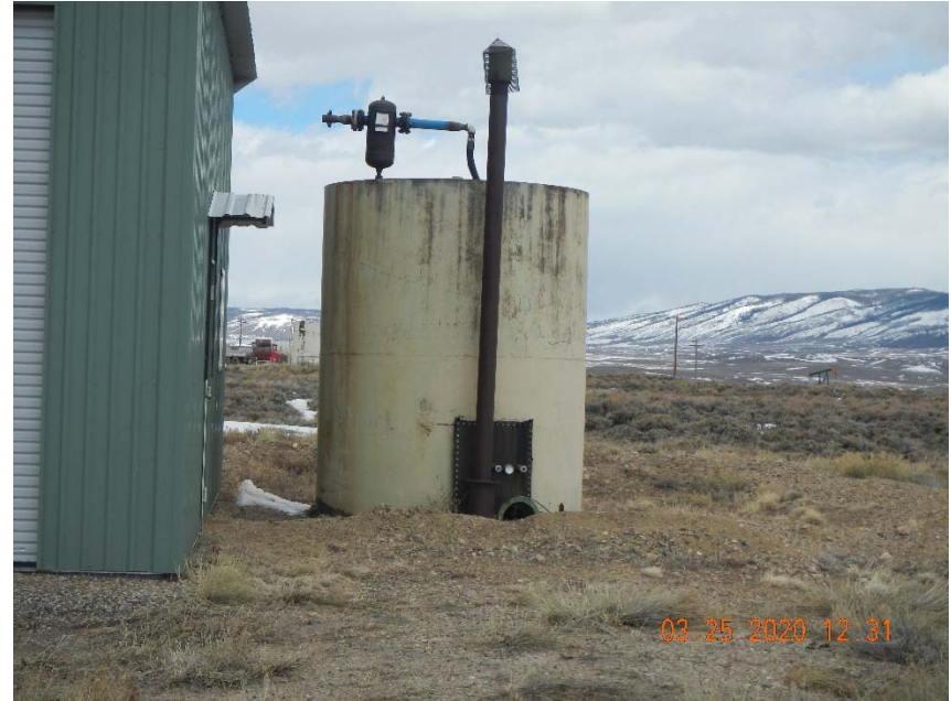
Photo 2. No label on tank.
