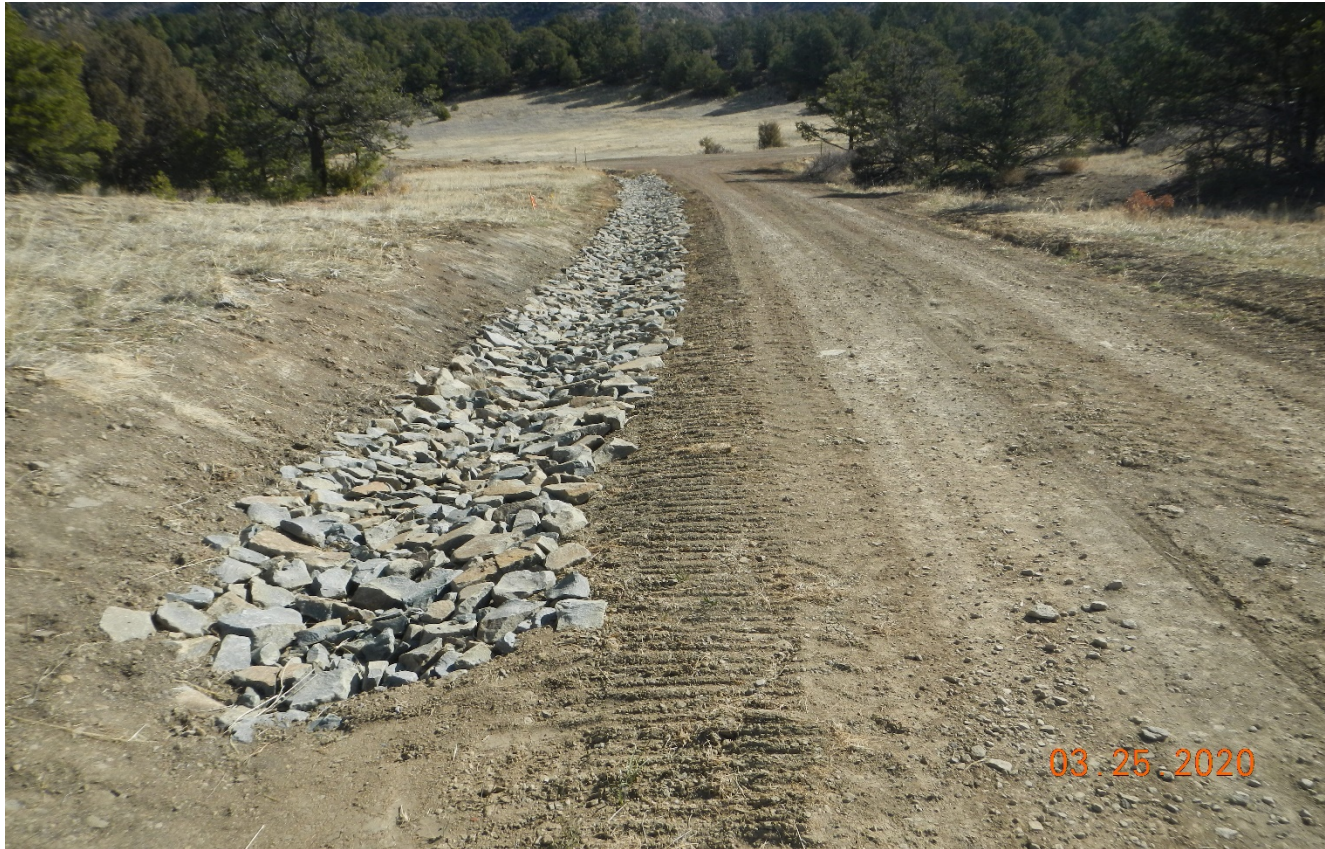
Photo 1. Rock rip/rap has been installed along the lease road as it ascends the hill.
