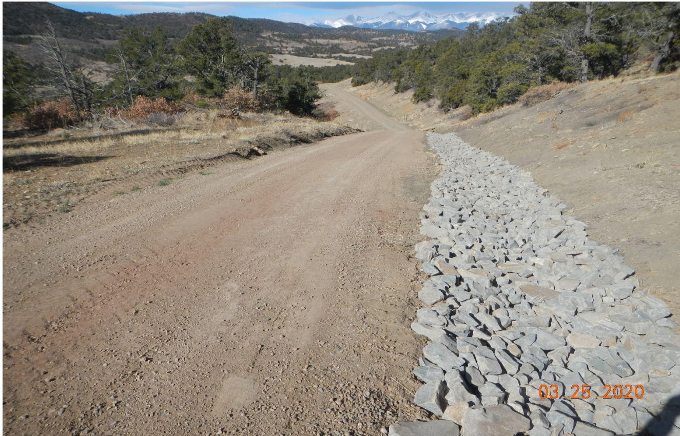
Photo 2. Facing west along the lease road. Rock rip/rap has been installed along the lease road as it descends the hill.
