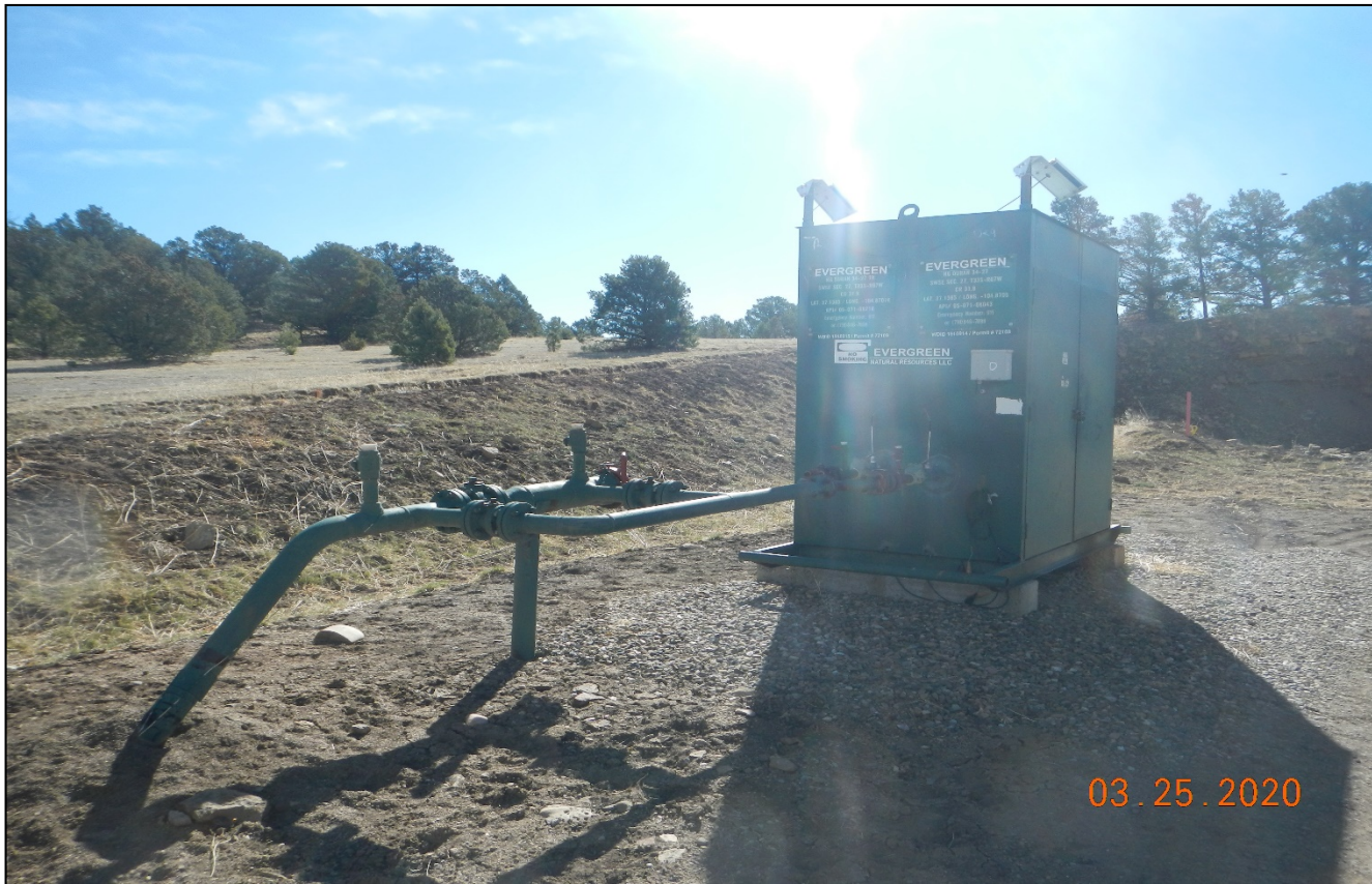
Photo 6. The well sign is posted at the meter shed.
