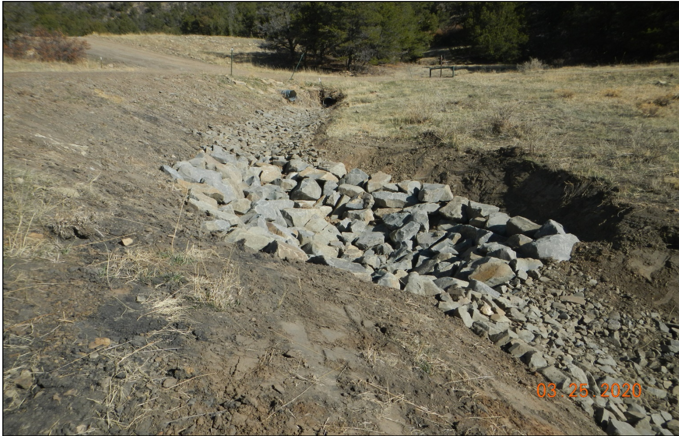
Photo 3. Culvert outlet protection and a rock sediment trap have been installed in drainage area.
