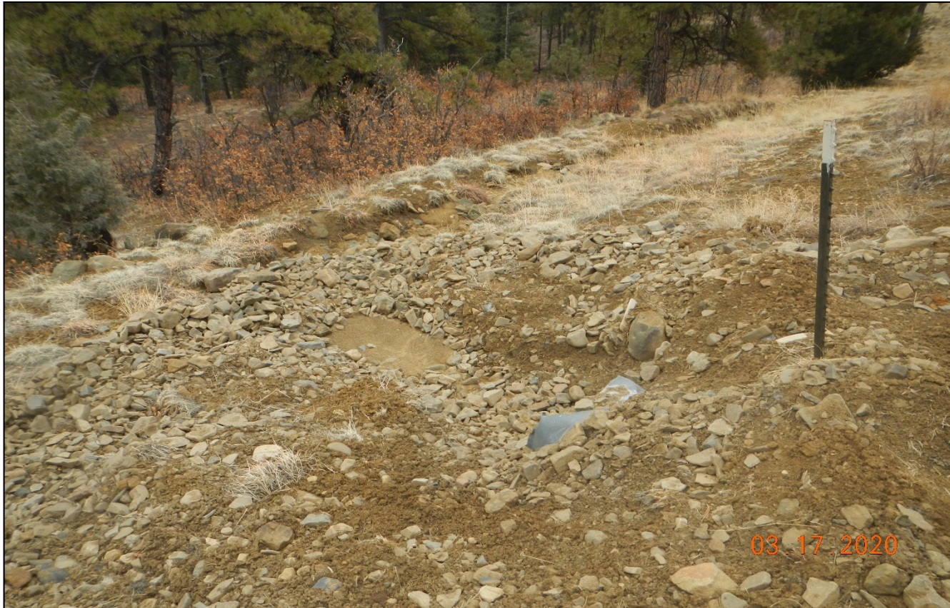
Photo 2. It appears rock rip/rap was placed at the culvert outlet and is capturing sediment. This may need to be cleaned at and enlarged.
