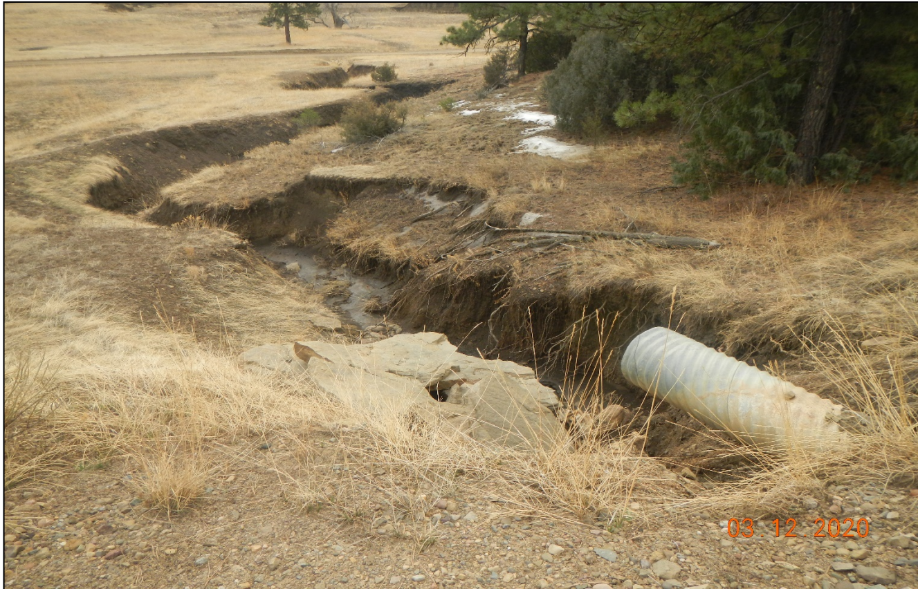
Photo 1. There is erosion occurring at this culvert outlet along the main road at Lat/Long:37.05979,-104.81561. No culvert outlet BMP to prevent erosion. Stormwater is being directed to this area from the road.
