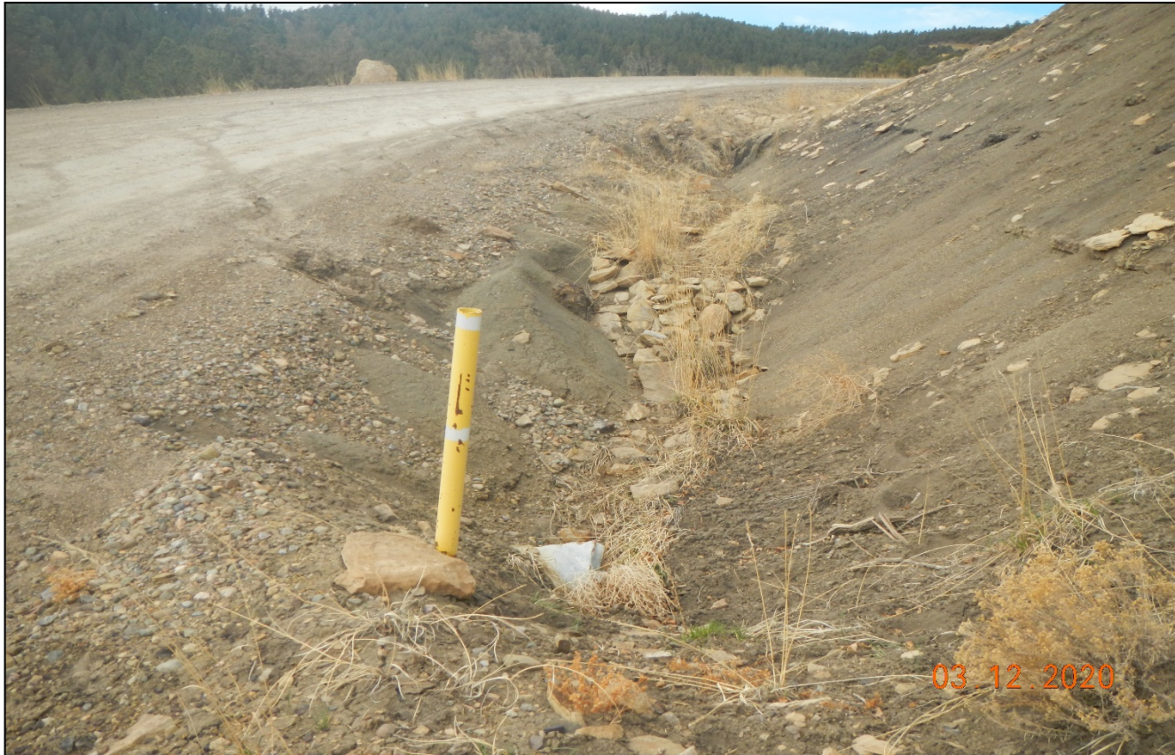
Photo 4. Erosion is occurring on the side of the road and this culvert has filled in with sediment at Lat/Long:37.0586,-104.81750.
