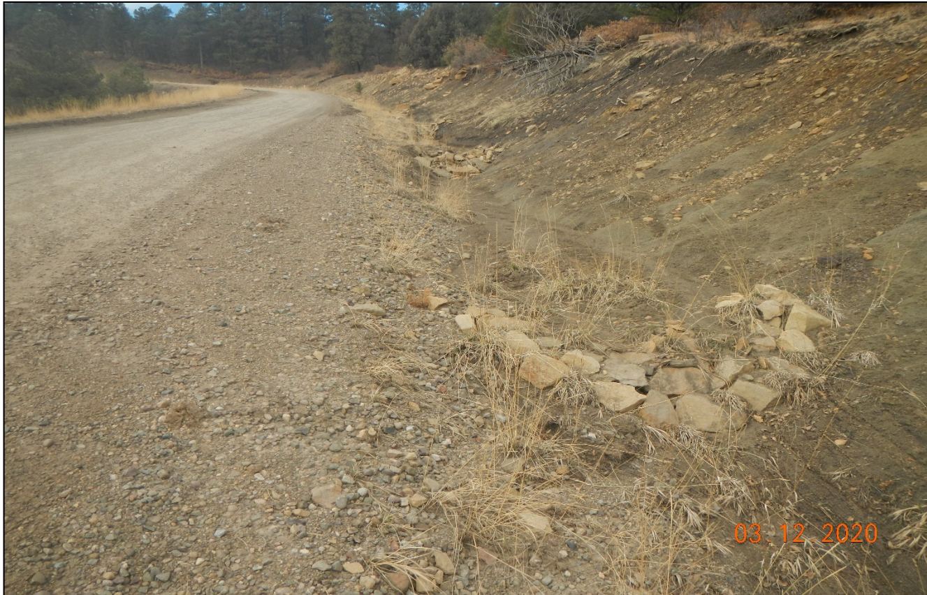
Photo 3. Erosion is occurring on the side of the road and rock check damns have filled up with sediment at Lat/Long:37.0586,-104.81750.
