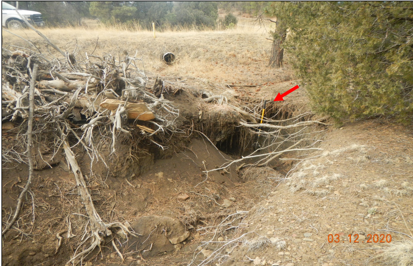
Photo 2. Further up the road there is erosion occurring from the culvert outlet along the main road at Lat/Long:37.05963,-104.81659. No culvert outlet BMP to prevent erosion. Red arrow points to 4.5 foot shovel placed in erosion gully.
