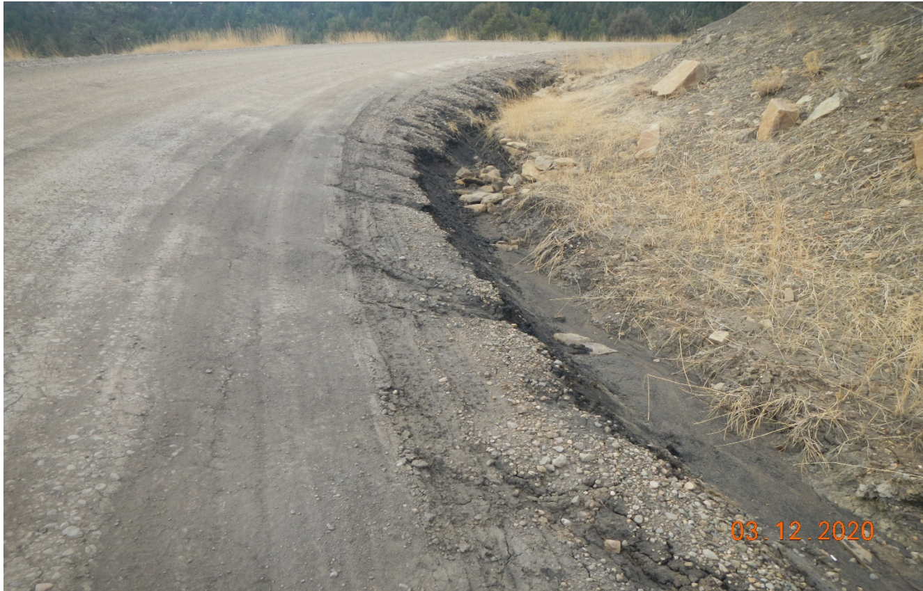
Photo 5. There is erosion occurring along the main road and no BMP's are installed to prevent erosion.
