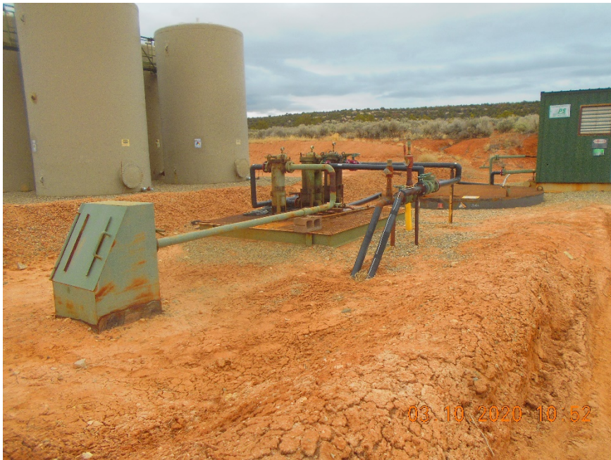
Loading station and Filter pod
