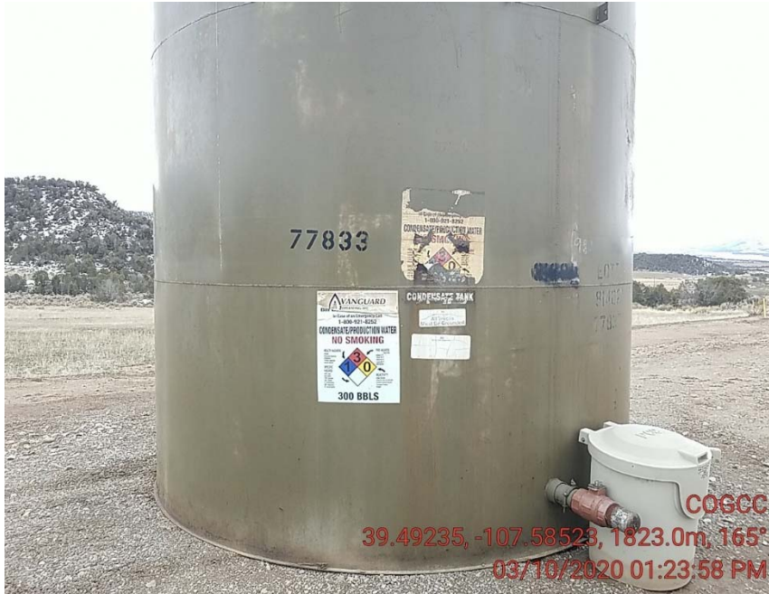
Un used equipment and improper labeling
