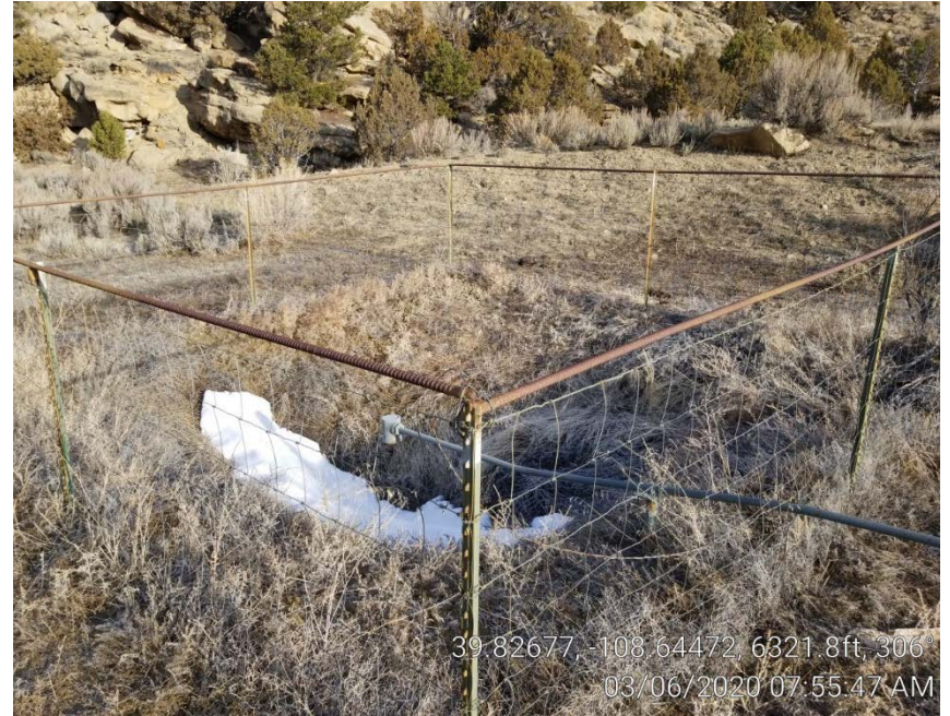
Photo 3. Weeds in gas meter pit.
