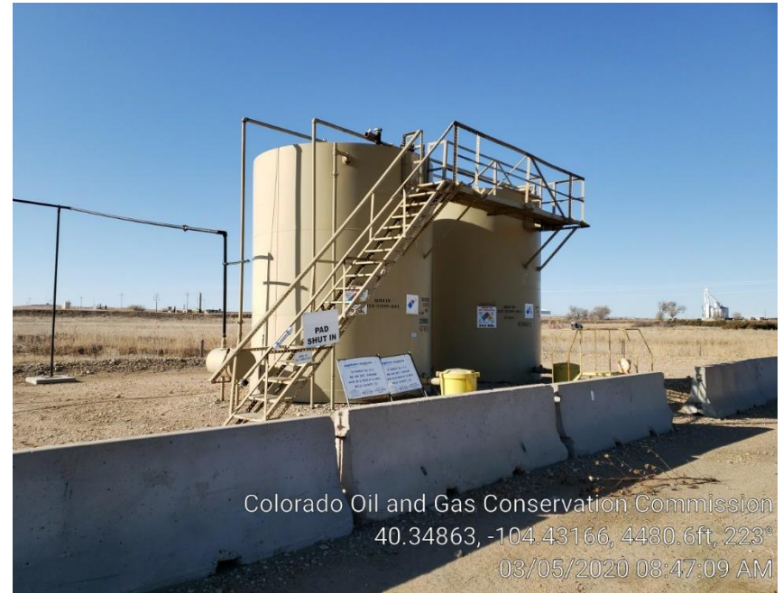
Photo #4 Tank Battery
