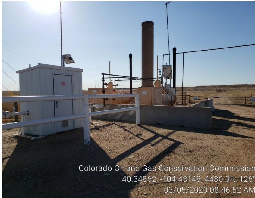
Photo #3 Separators, ECD & Meter Run
