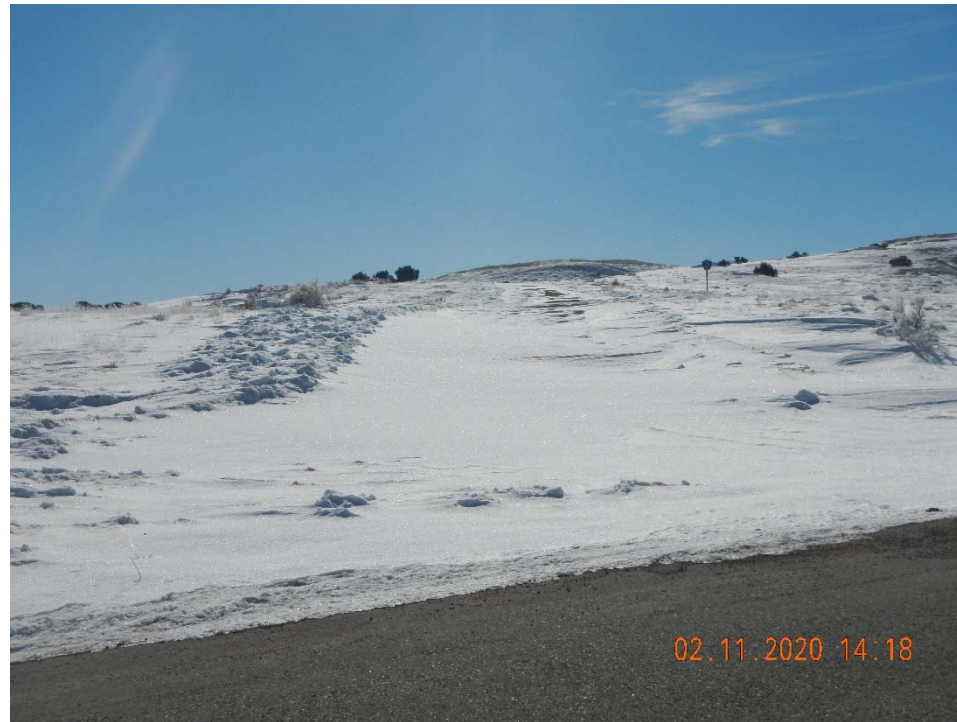
Photo 1. Access roads not maintained for winter.
